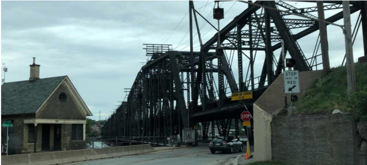
FIGURE 4-4: CRESCENT BRIDGE OVER THE MISSISSIPPI RIVER BETWEEN ROCK ISLAND AND DAVENPORT, IA
