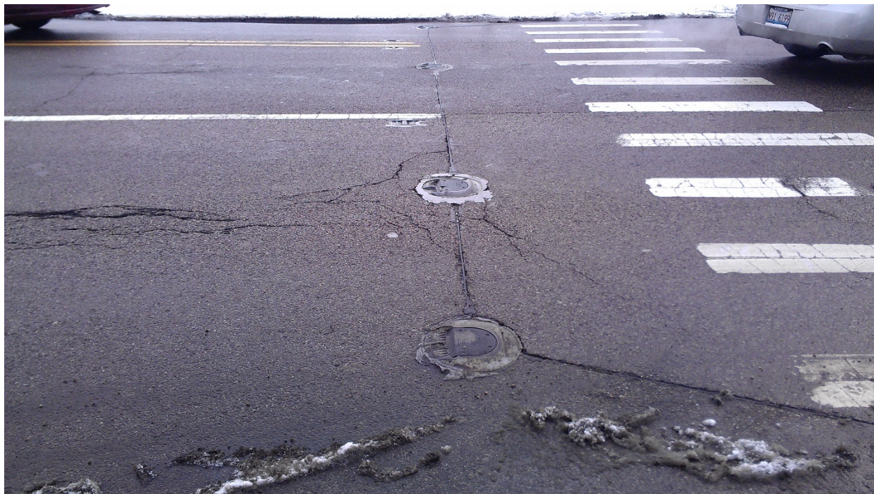
Figure 11 – Flush mounted IRWLs during the winter on Roosevelt Road (IDOT) in Oak Park, Illinois
