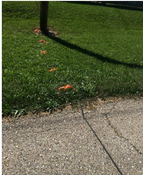
Figure 5 - Small cracks in widened shoulders along County Highway 56 (Rochester Road) from East Lake Shore Drive in Springfield, Illinois, to Ebel Drive in Rochester, Illinois. Timely maintenance of these cracks will increase the longevity of the paved shoulder and preserve riding surface.
