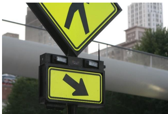
Figure 21 - Rectangular rapid flashing beacon lights
