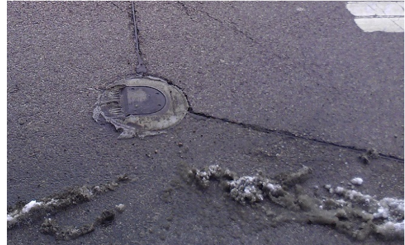
Figure 8 – In-roadway warning light during winter conditions, covered in road grime and salt, on Roosevelt Road (IDOT) in Oak Park, Illinois
