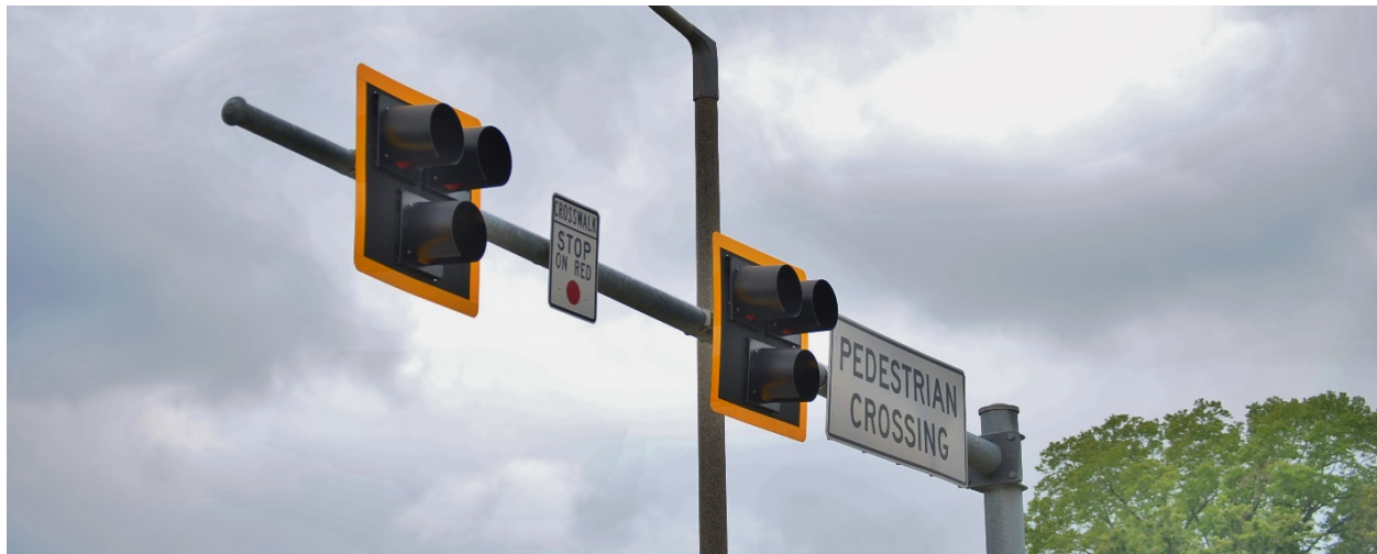
Figure 9 - PHB Signal in Pekin, Illinois.
