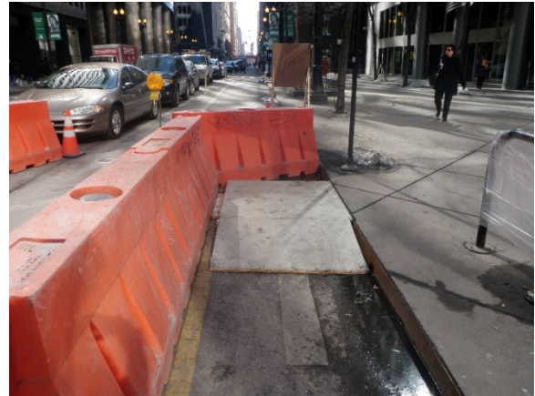
Figure 28 - Example maintenance of traffic that provides a temporary handicap accessible ramp for the pedestrian detour
