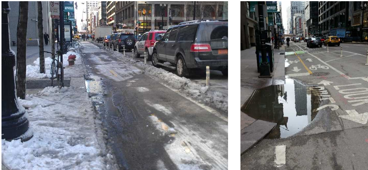
Figure 16 - Drainage issues resulting in ice forming on the Dearborn Street two-way separated bicycle lane in Chicago
