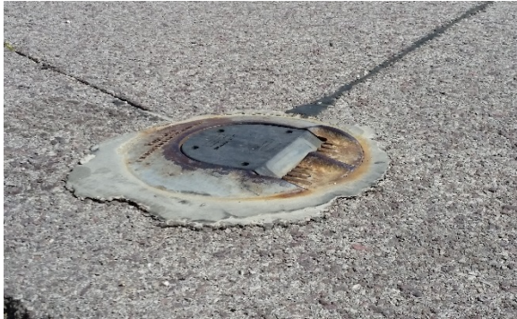
Figure 7 – In-roadway warning light during dry and sunny conditions, on Roosevelt Road (IDOT) in Oak Park, Illinois
