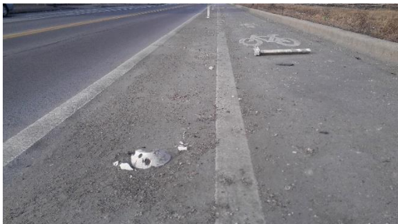
Figure 13 – Road grit and a broken bollard left from melting winter snow on the Vincennes buffered bicycle lane in Chicago
