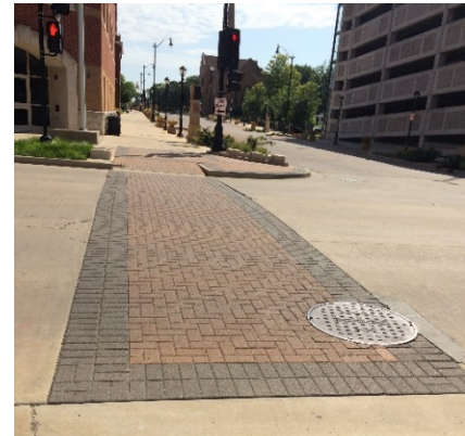
Figure 9 - Brick paved crosswalk in Springfield, Illinois. Not MUTCD compliant due to no white striping on traversing sides of crosswalk.
