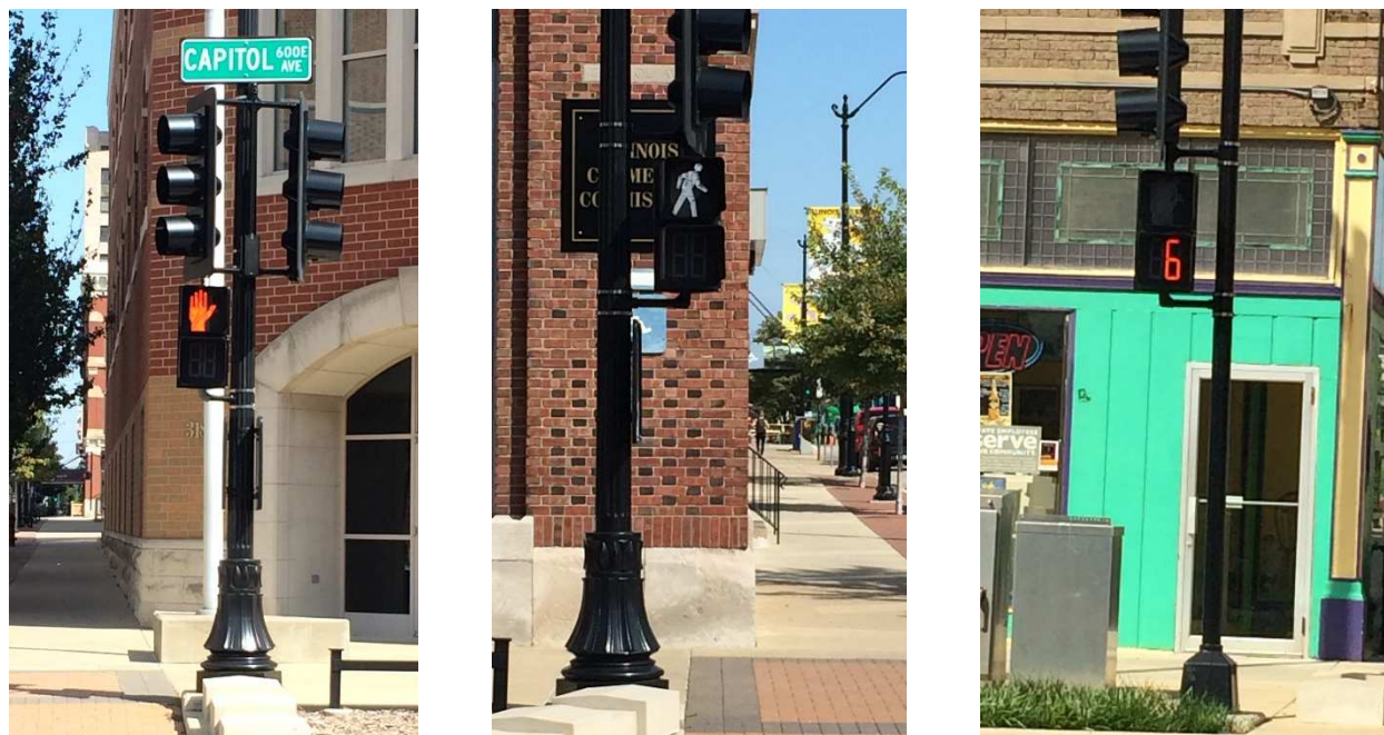
Figure 1 - Pedestrian signal heads in Springfield, Illinois, reflecting various indications (left to right: upraised hand (DON'T WALK), walking person (WALK), and countdown display indicating number of seconds remaining in the pedestrian change interval)
