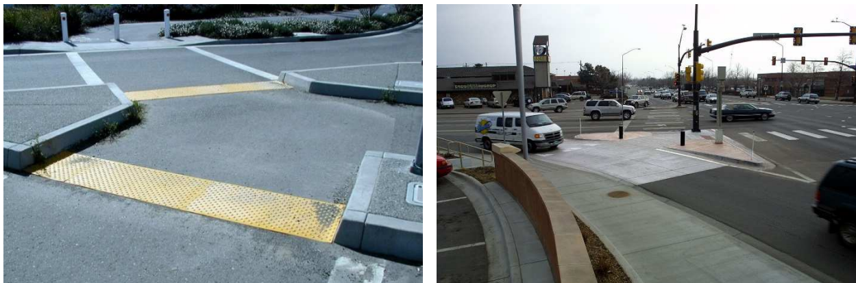
Figure 3 – Left: right turn corner island with a cut-through crossing and properly orientated detector pads. Right: right turn corner island with raised crosswalk and yield markings. Images: www.pedbikeimages.com / Dan Burden
