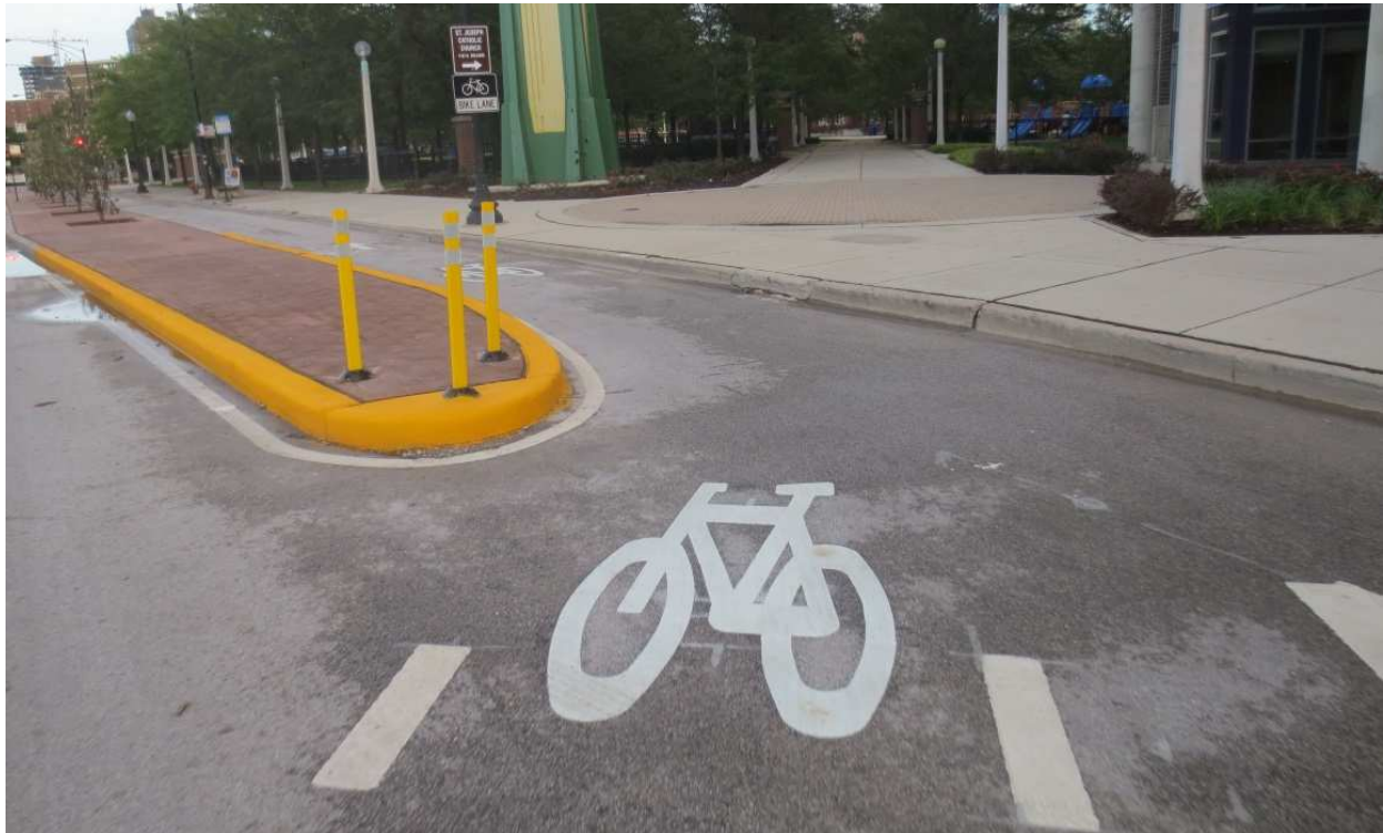
Figure 8 - Entrance to the curb separated bicycle lane on Division Street (a state route) in Chicago. The curb is painted yellow and installed with delineating posts.
