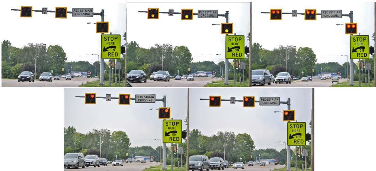
Figure 2 - Stages of PHB signal. Top image from Figure 4F-3 “Sequence for a Pedestrian Hybrid Beacon” in the 2009 MUTCD. Bottom images from a PHB in Pekin, Illinois.
