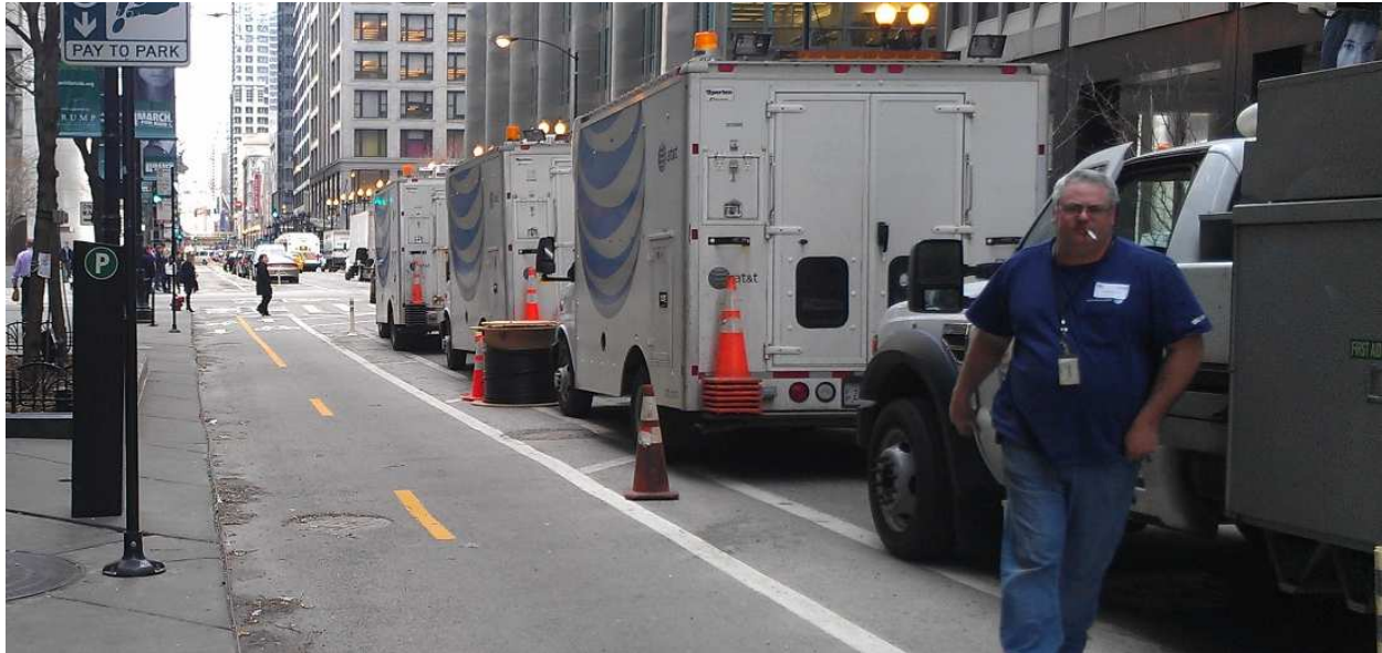
Figure 13 - AT&T crews preparing for utility work on the Dearborn Street two-way separated bicycle lane in Chicago
