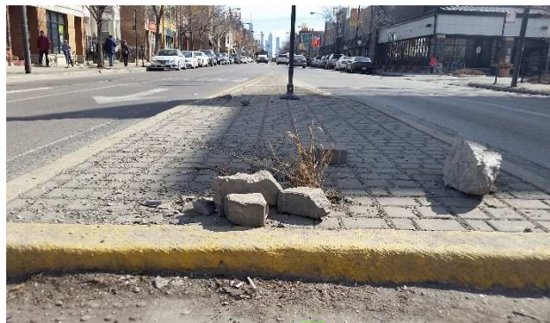
Figure 14 - Damaged median refuge island on Chicago Avenue and Hoyne Avenue in Chicago
