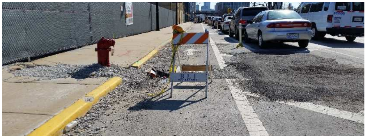
Figure 12 - A one-way separated bicycle lane blocked by utility construction along Jackson Street in Chicago
