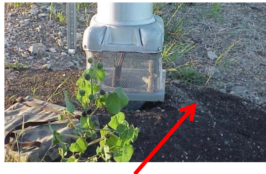
Unacceptable Does not meet 4" rule across a 60 inch chord.
