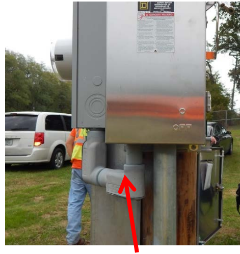
Acceptable RGC with rusted threads should be cleaned and treated with galvanizing compound or replaced.
