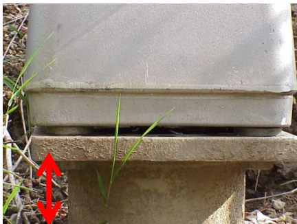
Unacceptable Violates the 4" rule, installed too far above grade.
