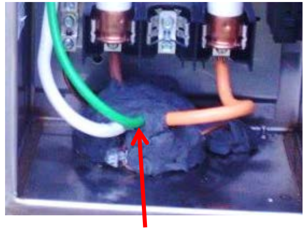
Acceptable Pliable waterproof material such as duct seal should be applied to all conduit entries.
