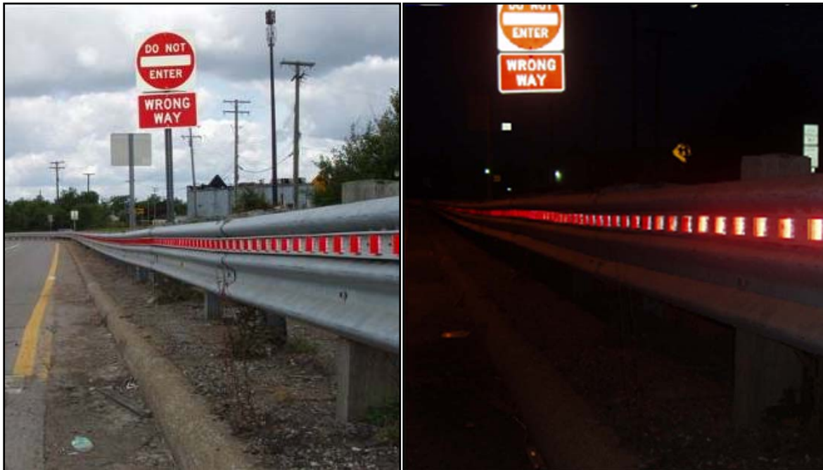
Figure 2-16. Barrier delineators visible while traveling in the wrong direction (Morena and Ault 2013).
