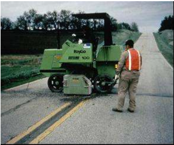
Step 1. Pre-overlay repair & surface preparation. Localized areas of distress are repaired prior to overlay placement.
