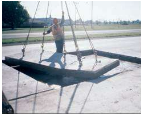
Step 2. Concrete removal. Removal of slab material is best accomplished using the lift-out method or by breakout.
