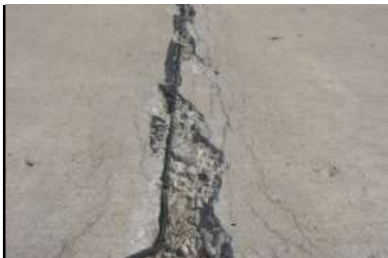
Severe D-Cracking - A well defined cracking pattern with a significant amount of loose or missing material.
