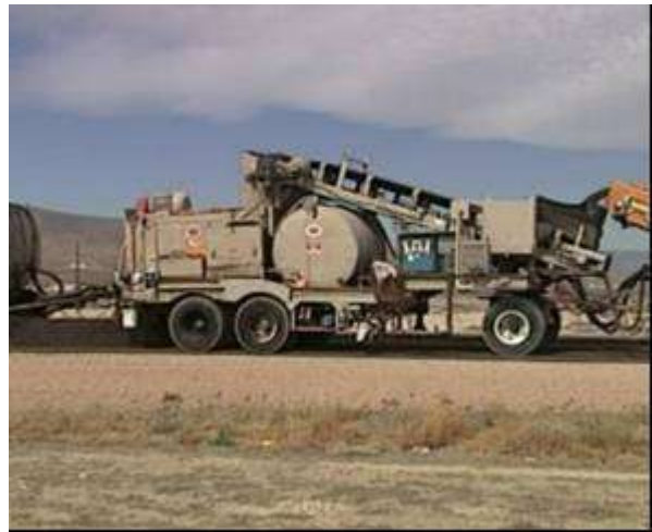
Step 2. Mix recycling. Next, the milled material is crushed, sized, mixed with recycling additives.
