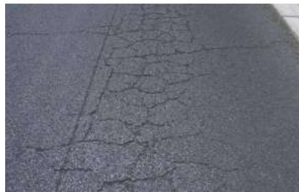
Moderate Alligator Cracking - Cracks are interconnected and may be slightly spalled, but are stable.
