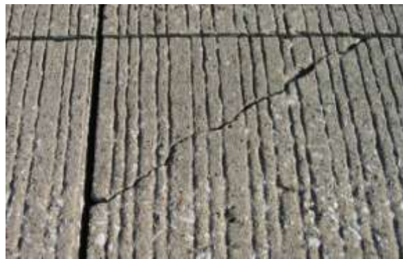
Light Corner Breaks - Crack is hairline and unspalled; the resulting corner piece is not cracked or shows no movement under load.
