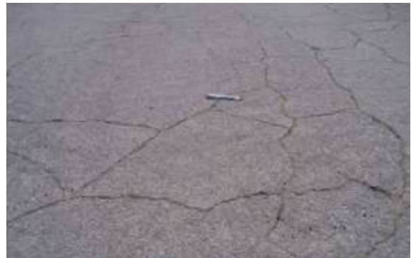
Moderate Block Cracking – Cracks have opened up, exhibit a small amount of spalling, or have adjacent random light cracking.
