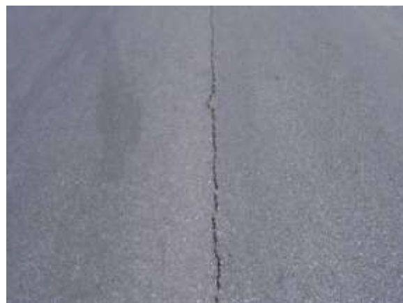
Light L&T Cracking - Tight cracks or sealed cracks with the filler in good condition.
