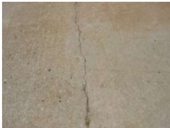
Light Transverse Cracking - Tight cracks with little or no spalling and no faulting.
