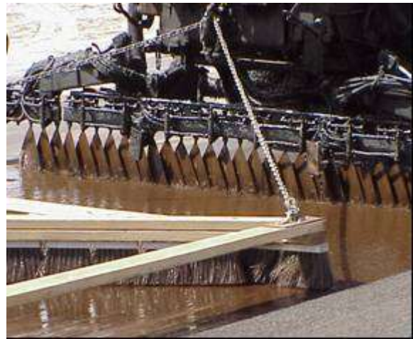
Step 2. Emulsion application and drag-brooming. Drag-brooming is used to work emulsion into cracks and surface voids.
