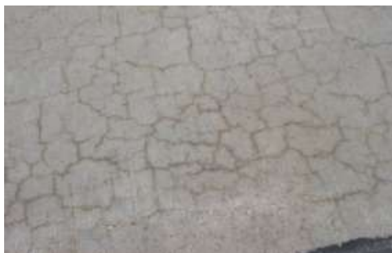
Light Surface Distress - Very clear cracking pattern on the surface, where cracks appear tight and shallow; no scaling.
