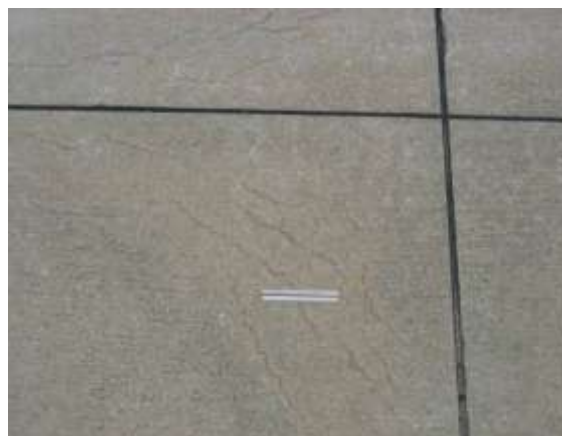
Light D-Cracking - Tight cracks with no loose or missing pieces and no patching in the affected area.
