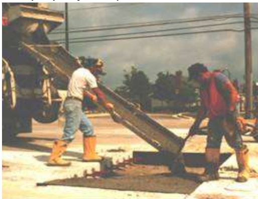
Step 5. Material placement. Conventional PCC material is most common for full-depth repairs.
