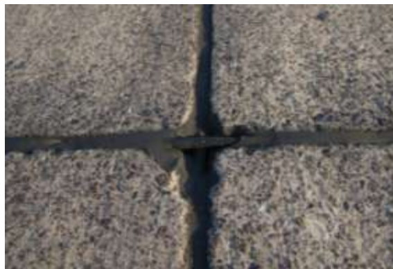
Moderate Joint Seal Damage - Portions of the sealant are missing, oxidized (no longer pliable), split, or have lost adherence.
