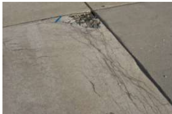
Moderate D-Cracking - Well defined cracks, with a few small loose pieces.
