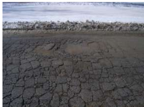
Severe Alligator Cracking - Cracks are wider and pieces are spalled and show movement under traffic loads.
