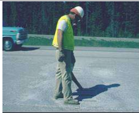
Step 3 & 4. Sandblasting and cleaning. Slots are sandblasted and cleaned in preparation for dowel bars.
