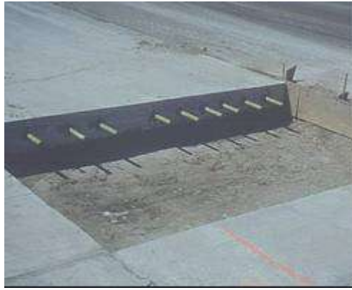
Step 4. Load transfer provision. Proper restoration of load transfer should be considered.
