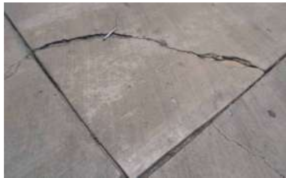
Moderate Corner Breaks - Crack has some spalling and the corner piece is intact and has little or no movement under load.
