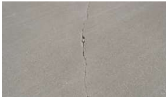
Light Longitudinal Cracking - Tight cracks with little or no spalling.
