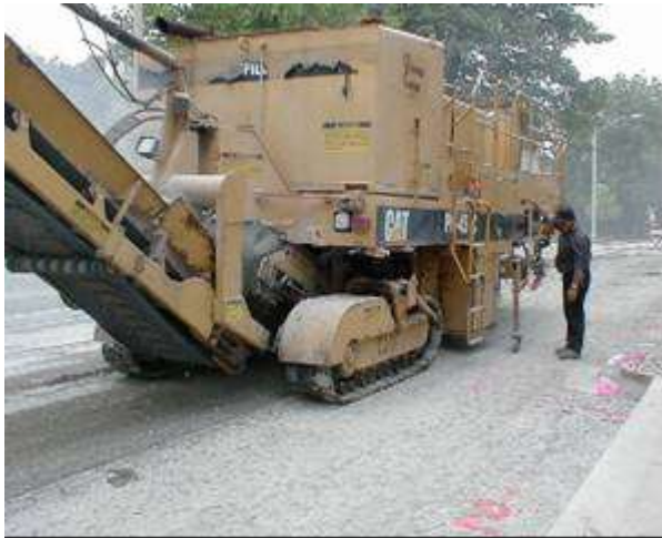
Step 1 & 2. Pre-overlay repair & milling and cleaning. Localized areas of distress are repaired prior to overlay placement. The surface is milled to remove rutting and restore profile prior to PCC placement.
