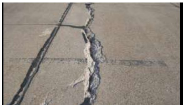
Severe Longitudinal Cracking - Cracks that exhibit movement accompanied by discernable spalling.
