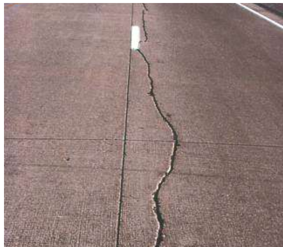
Moderate Longitudinal Cracking - Wider cracks with some spalling.
