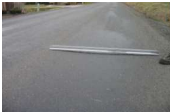
Light Rutting - Rut depth visible, approximately less than ½ inch (12.7 mm) in a given location.
