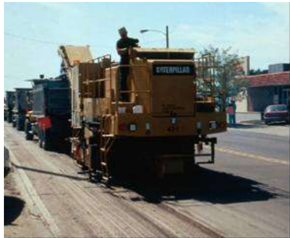
Step 2. Milling. If necessary, milling is used to remove distress and promote bonding with the existing surface.
