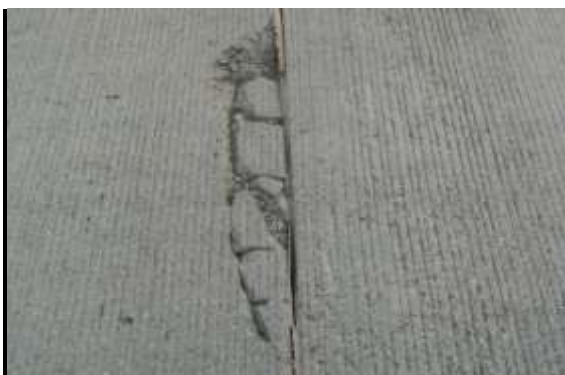
Severe Spalling - Considerable wear and loss of material at the joint or crack; ride quality is affected.
