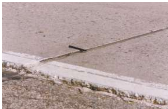
Moderate Faulting - Faulting measures approximately ¼ inch to ½ inch (6.4 mm and 12.7 mm) at a given location.
