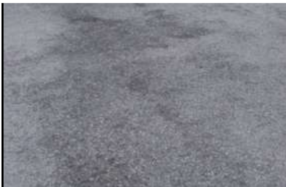
Severe Weathering/Raveling - Considerable aggregate loss resulting in an overall rough pavement surface with pitted/eroded areas.
