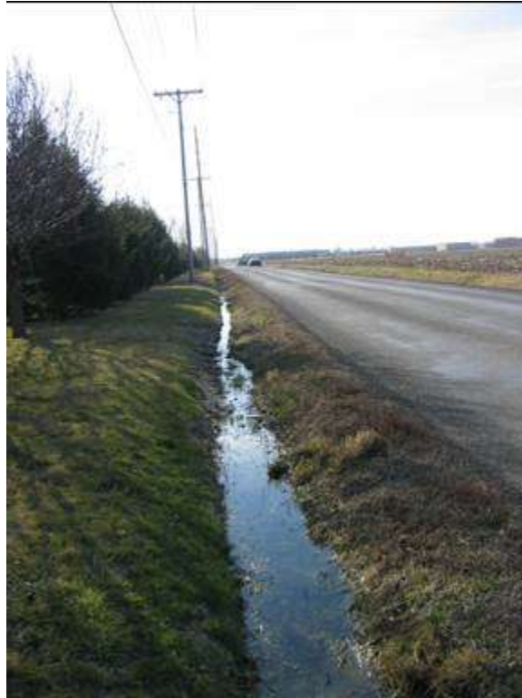
Drainage Preservation. This photo shows an example of a ditch with obstructed flow.
