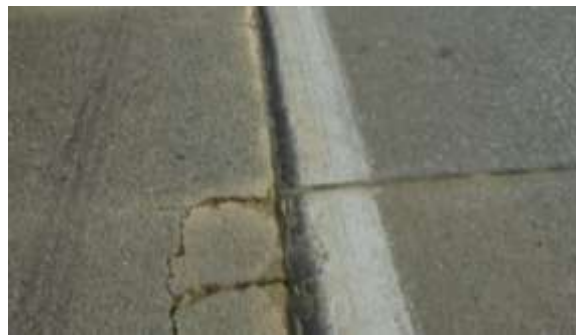
Light Pumping - Small areas of staining visible.
