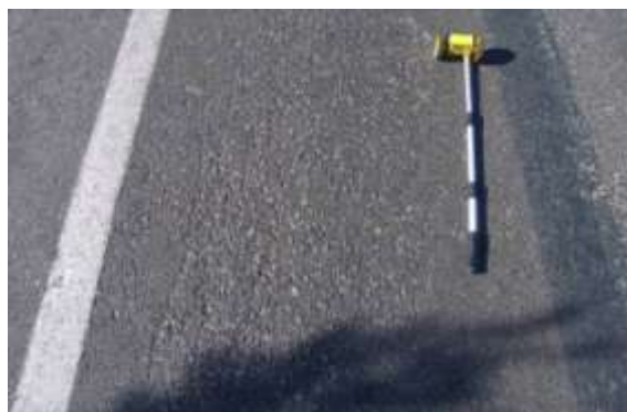
Light Weathering/Raveling - Some aggregate loss from the pavement surface with little or no pitting.
