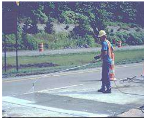
Steps 6 & 7. Texturing & Curing. The final steps include texturing and providing adequate curing.
