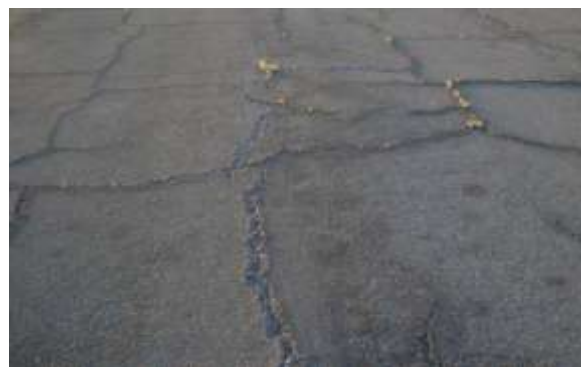
Severe Block Cracking – Cracks are wide, have significant spalling, or are accompanied by adjacent moderate severity random cracking.
