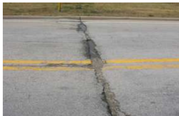
Severe L&T Cracking - Cracks are wide, have significant spalling, or are accompanied by adjacent moderate severity random cracking.
