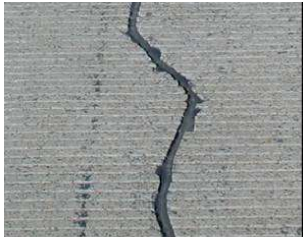
Step 4. Application of sealant. The last step is to place the sealant in the refaced crack per governing specifications.
