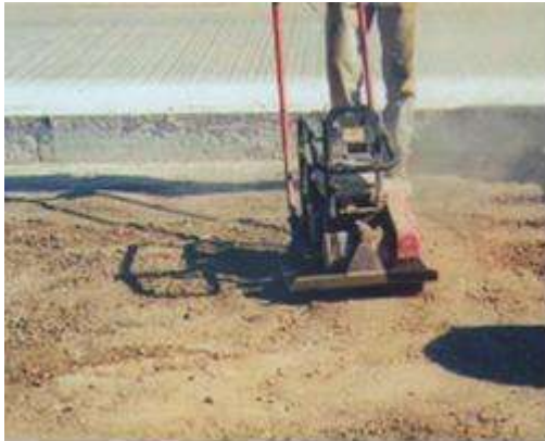
Step 3. Repair area preparation. It is important that the repair area be dry and properly compacted.
