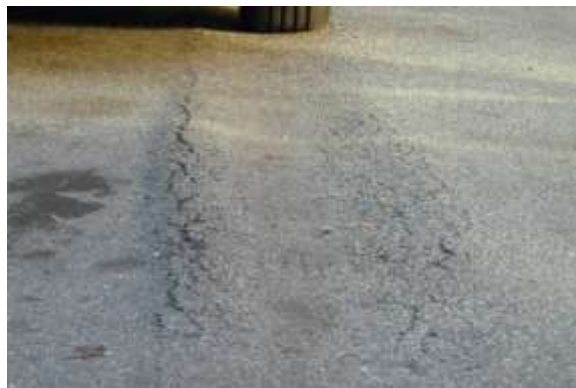
Severe Rutting - Rut depth greater than approximately 1 inch (25.4 mm) in a given location.
