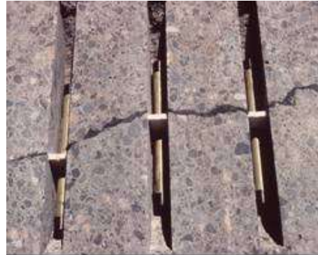
Step 6. Dowel bar placement. Dowels are placed parallel to the direction of traffic and at mid-slab.
