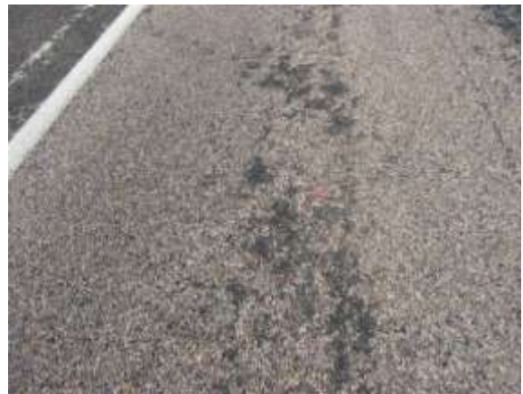
Light Bleeding – Small or isolated areas where asphalt material has pooled on the pavement surface.
