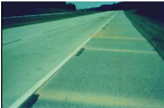
Severe Pumping - Excessive amounts of staining. Additional indications may include faulting or the erosion of shoulder pavement from applied pumping forces.
