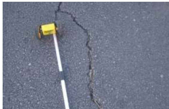
Moderate L&T Cracking - Cracks have opened up, exhibit a small amount of spalling, or have adjacent random light cracking.
