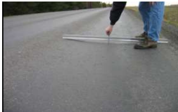
Moderate Rutting - Rut depth approximately between ½ inch and 1 inch (12.7 mm and 25.4 mm) in a given location.
