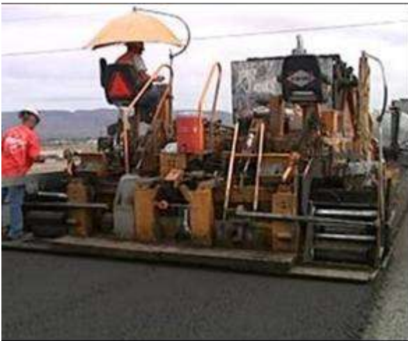
Step 3. Laydown. Conventional paving equipment is used to place the recycled material.
