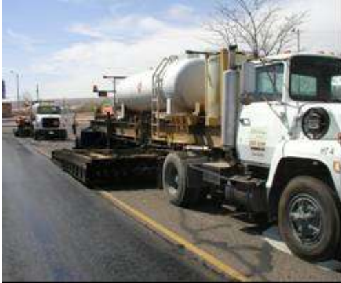
Step 1. Heating the surface. The surface is heated to soften the existing material.
