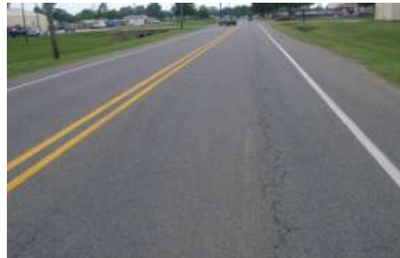
Light Alligator Cracking - A longitudinal crack or a series of parallel longitudinal cracks with little or no interconnection.
