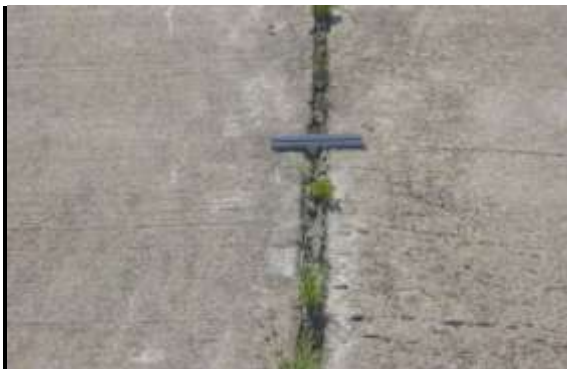
Severe Joint Seal Damage - Sealant is mostly missing, oxidized (no longer pliable), split, or is lost all adherence; sealant is no longer performing its intended function.
