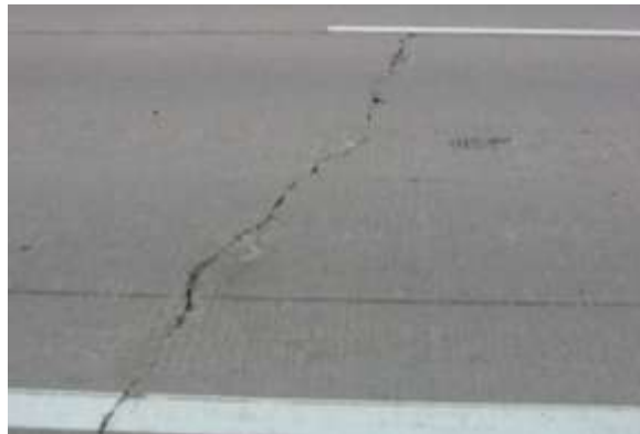
Moderate Transverse Cracking - Wider cracks with some spalling or faulting.
