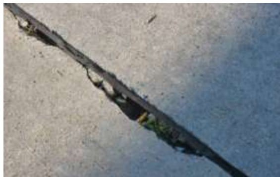
Moderate Spalling - Shallow but discernable wear at the joint or crack, with loose pieces that can be removed easily or are missing.
