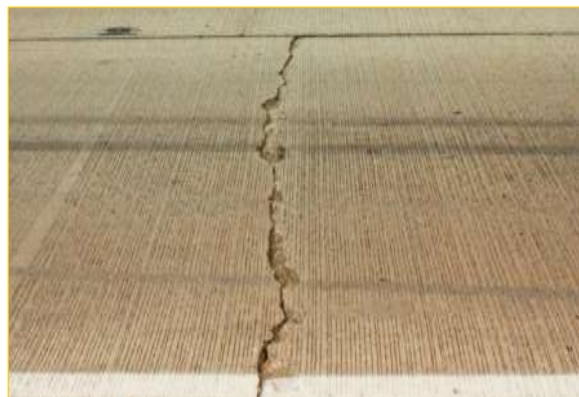
Severe Transverse Cracking - Cracks that exhibit movement accompanied by discernable spalling or faulting.
