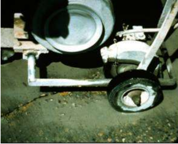
Step 1. Crack refacing. Small crack saws are used to reface cracks and create a reservoir for the sealant.
