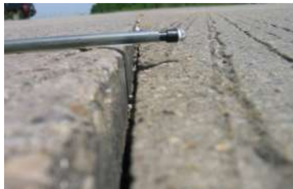
Severe Faulting - Faulting is greater than approximately ½ inch (12.7 mm) at a given location.
