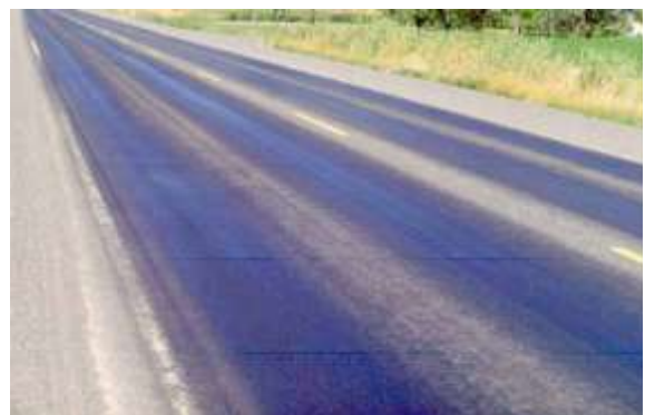
Severe Bleeding – Bleeding covers much of the pavement surface and is relatively thick.
