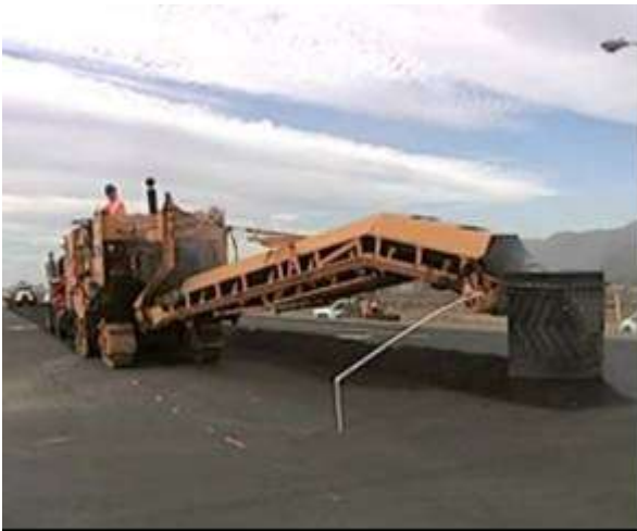
Step 1. Pulverization. In a multi-unit train, the pavement material is first milled and placed in a windrow.
