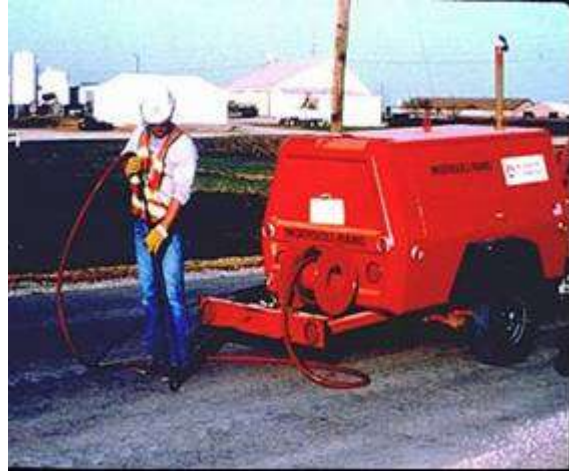
Step 2. Cleaning. Cracks must be clean and dry to enhance sealant bonding.
