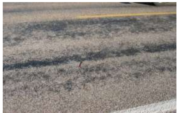
Moderate Bleeding – Bleeding is apparent over large or continuous areas of the pavement surface.
