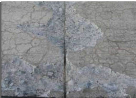
Severe Surface Distress - Extensive material loss (scaling).
