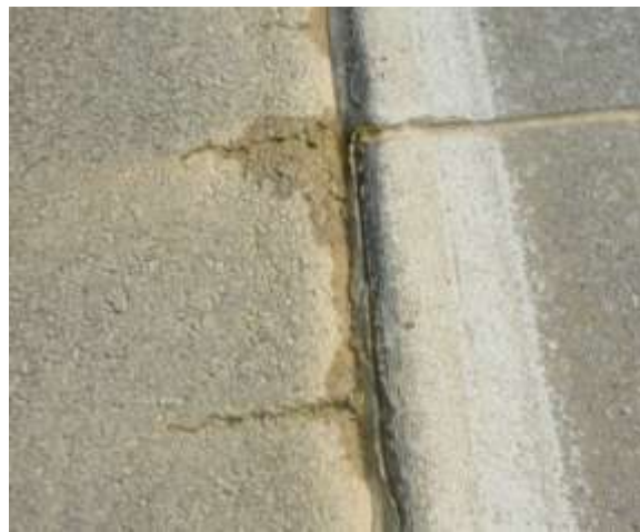
Moderate Pumping - Visible staining on the pavement surface.
