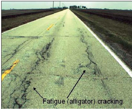
Figure 1. Fatigue cracking of the AC surface due to heavy, repeated wheel loads on CR 9.
