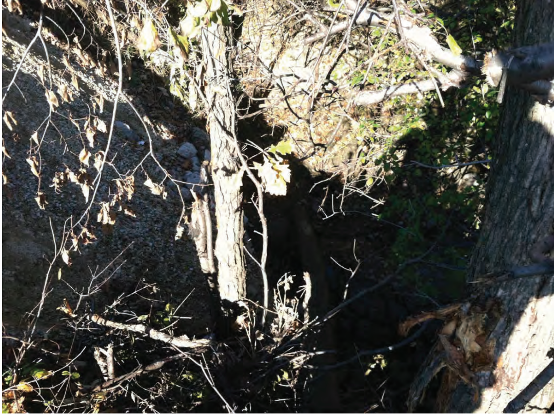
3. Looking North on River Road (Aggregate Fill Added by IDOT)
