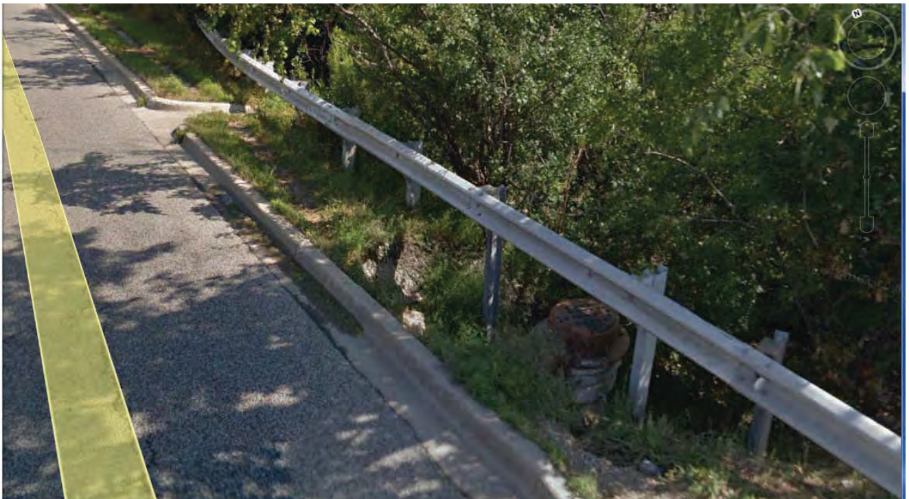
2. Looking Northeast at Drainage Structure on River Road (Before Gravel Fill Added)
