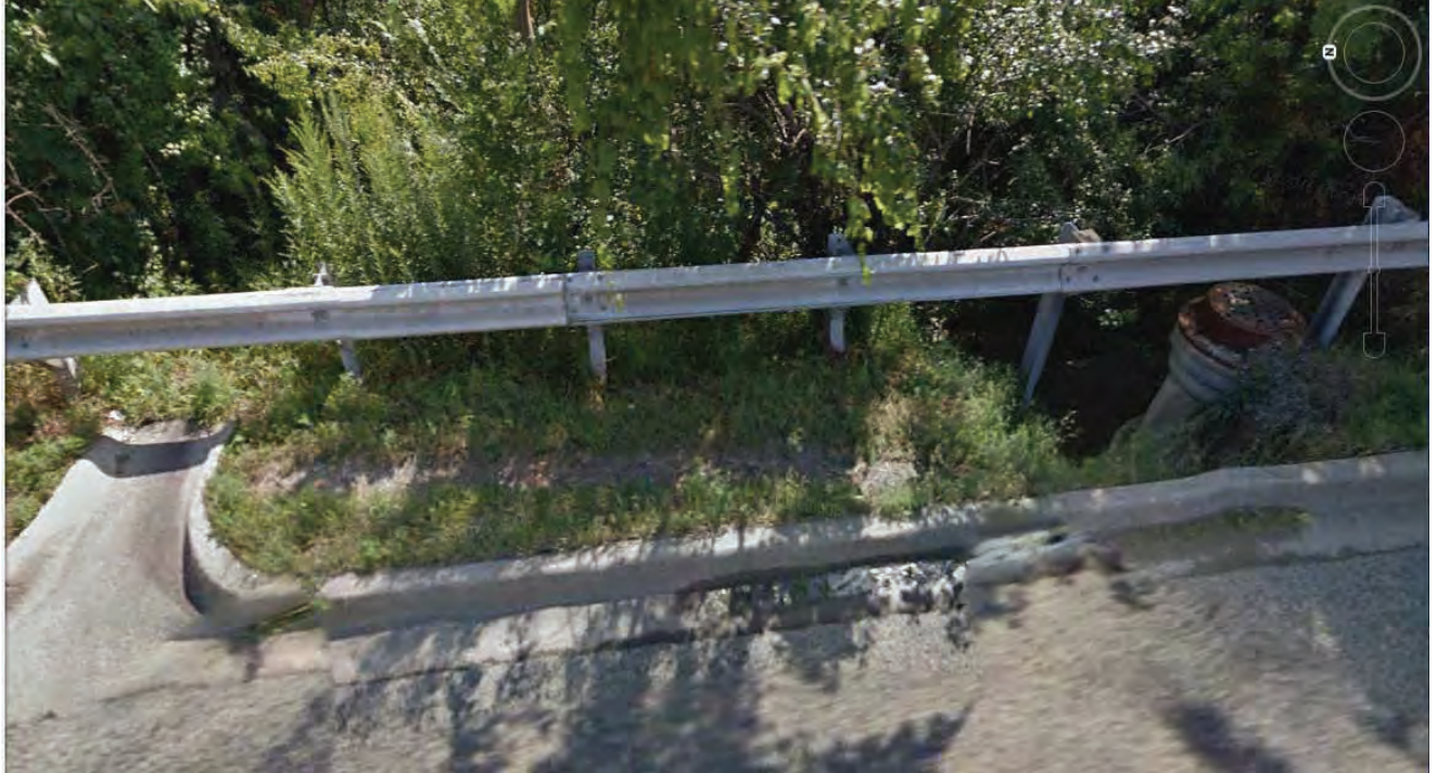
1. West of Culvert Looking East on River Road (Before Gravel Fill Added)
