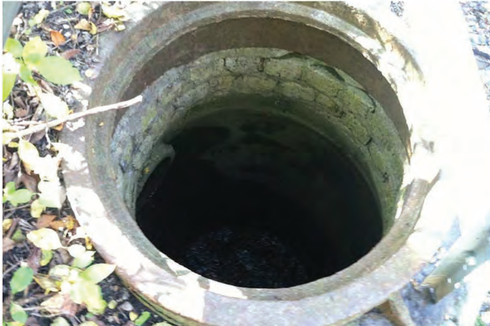
3c. FPCC manhole missing lid
