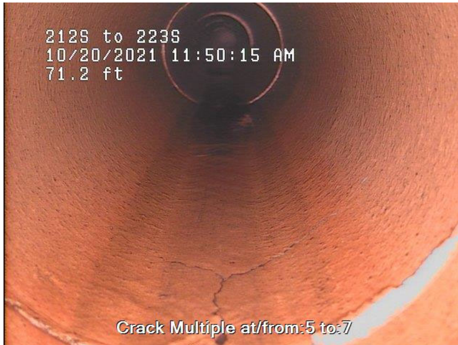
Example: Multiple Cracks
