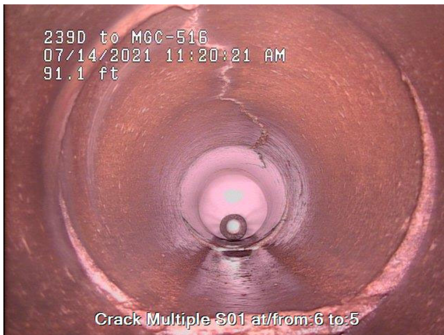
Example: Multiple Cracks
