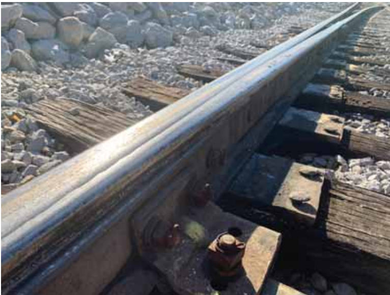
ABRASIVE SWITCH POINT WEAR WITH LIPPING ONTO STOCK RAIL
