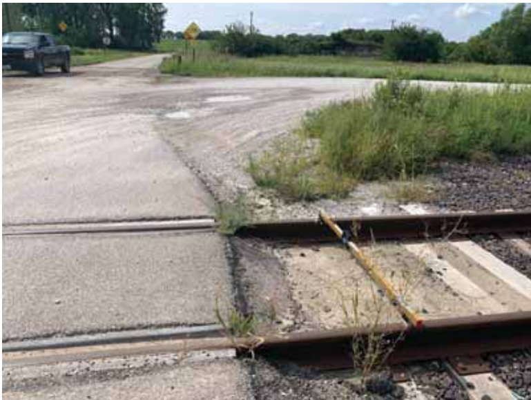
FOULED TRACK BALLAST AND LACK OF POSITIVE DRAINAGE
