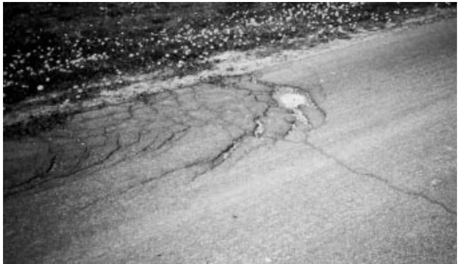
► Crescent-shaped cracks characteristic of slippage.
