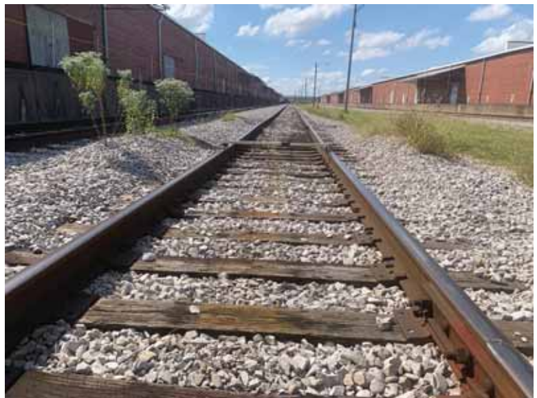
PROFILE DIP FROM SUBGRADE INSTABILITY HEAVING TRACK BALLAST SHOULDERS
