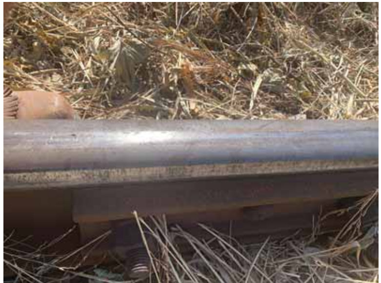
EXCESSIVE WEAR ON GAUGE SIDE OF RAIL
