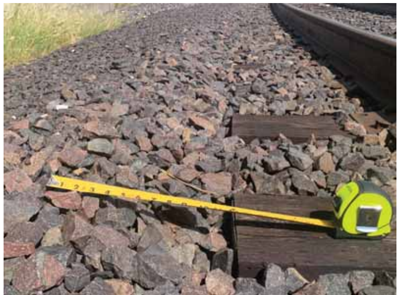
LATERAL TRACK MOVEMENT HEAVING BALLAST SHOULDERS
