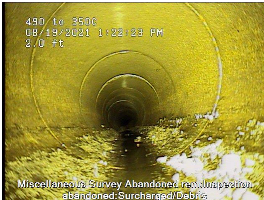
Example: Surcharge Debris
