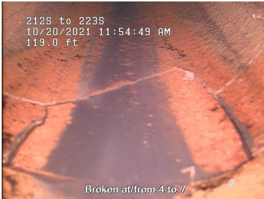
Example: Broken Pipe
