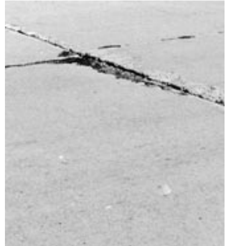
▼ Transverse joint has slight faulting and spalling.
