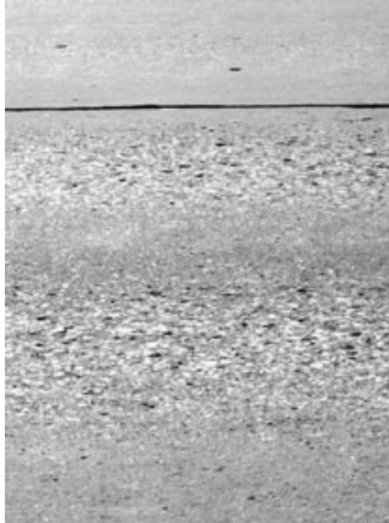
▶ Surface mortar worn away exposing larger aggregate. Accidents or friction testing may indicate a slippery surface in need of improved texture.
