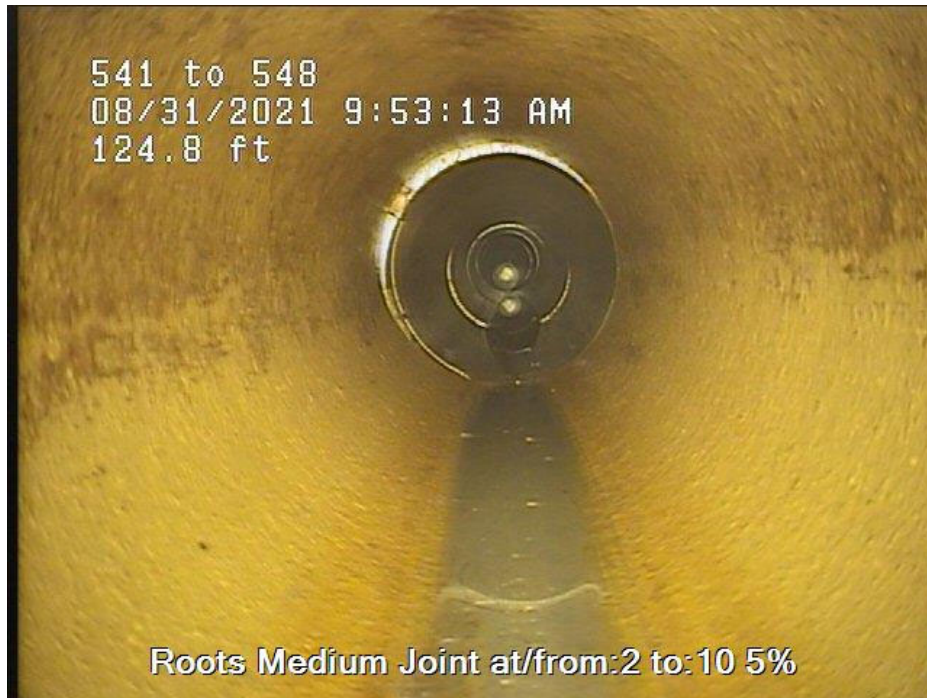
Example: Root Infiltration
