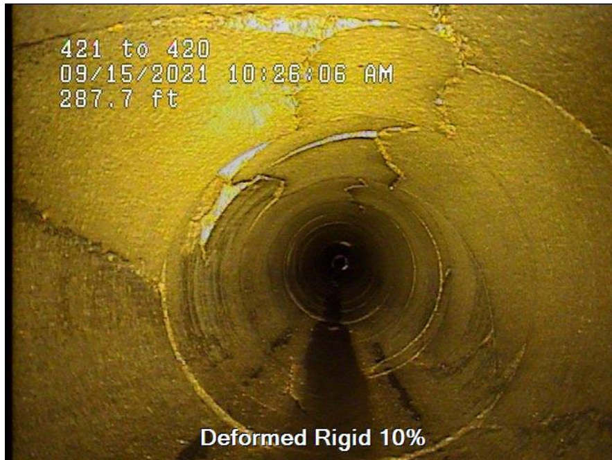
Example: Deformed Pipe (Rigid)
