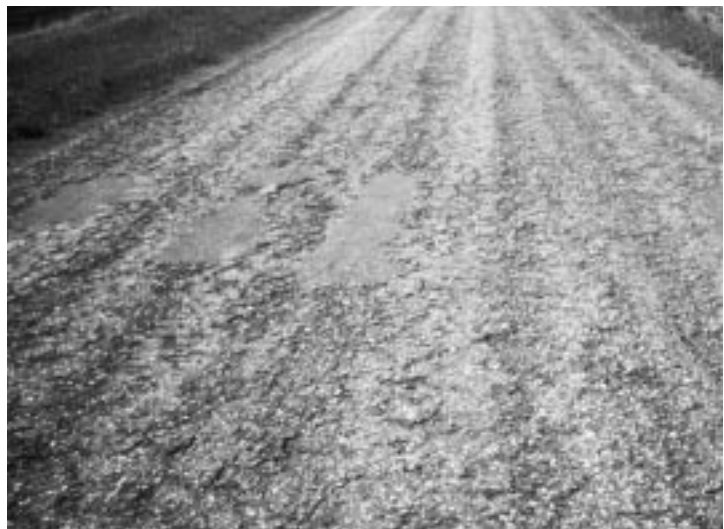
◀ Severe raveling and loss of surface material.
