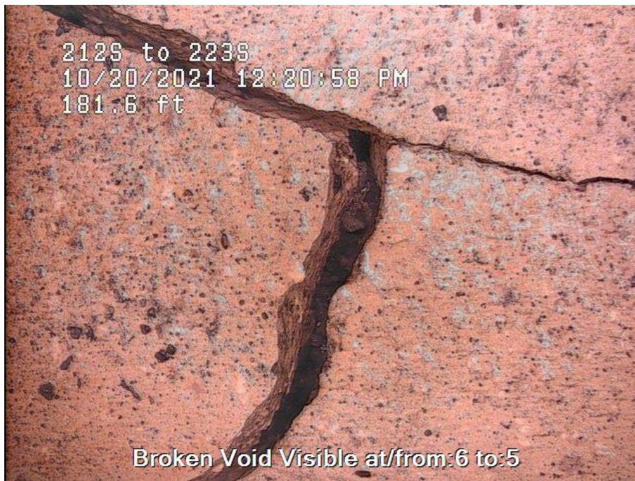
Example: Broken Pipe – Void Visible
