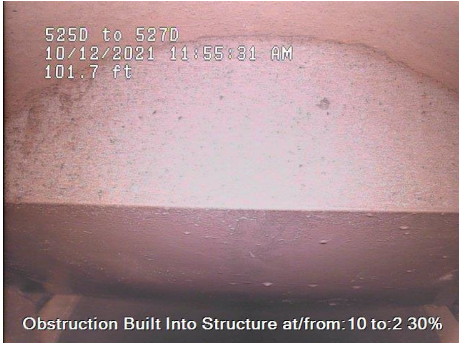
Example: Obstruction Built into Structure
