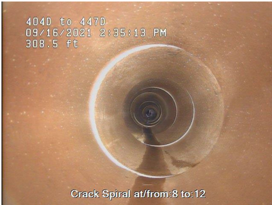
Example: Spiral Crack
