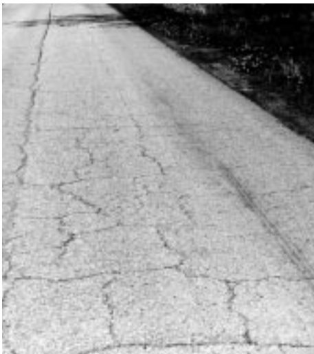
▲ Extensive block cracking in an irregular pattern.
