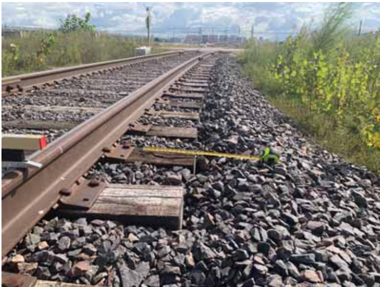
LATERAL MOVEMENT WITH BALLAST GAP AT TIE ENDS
