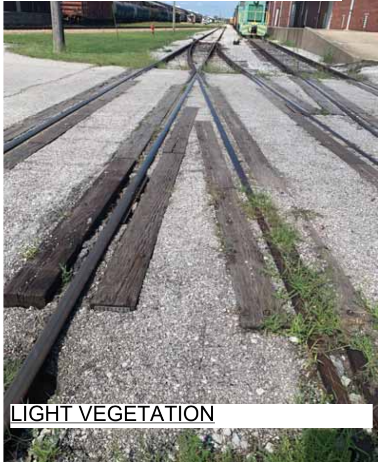
PAVEMENT SETTLEMENT ALONG GRADE CROSSING SURFACE
