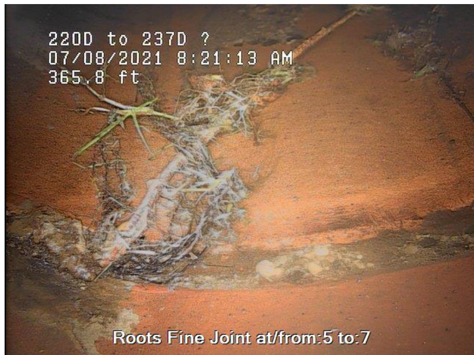
Example: Root Infiltration
