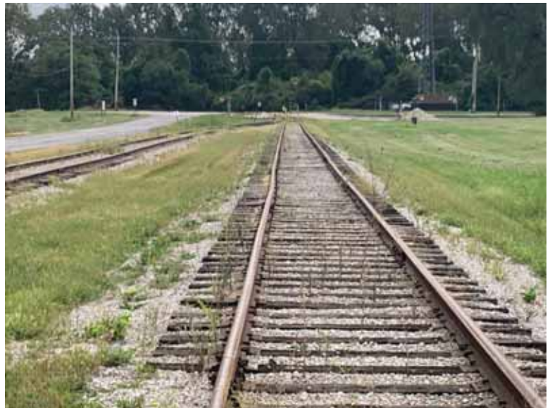
TRACK MISALIGNMENT WITH SHALLOW TIE CRIBS
