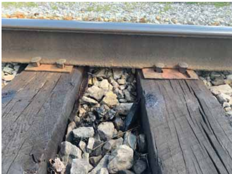
WEB AND BASE CORROSION OF SINGLE SHOULDER TIE PLATES
