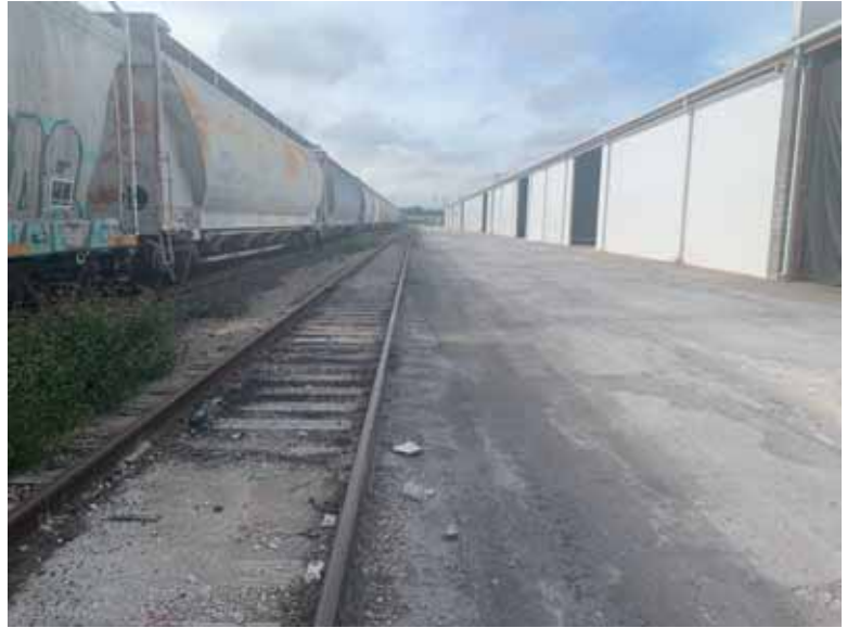
FOULED TRACK BALLAST FROM LACK OF ADEQUATE DRAINAGE
