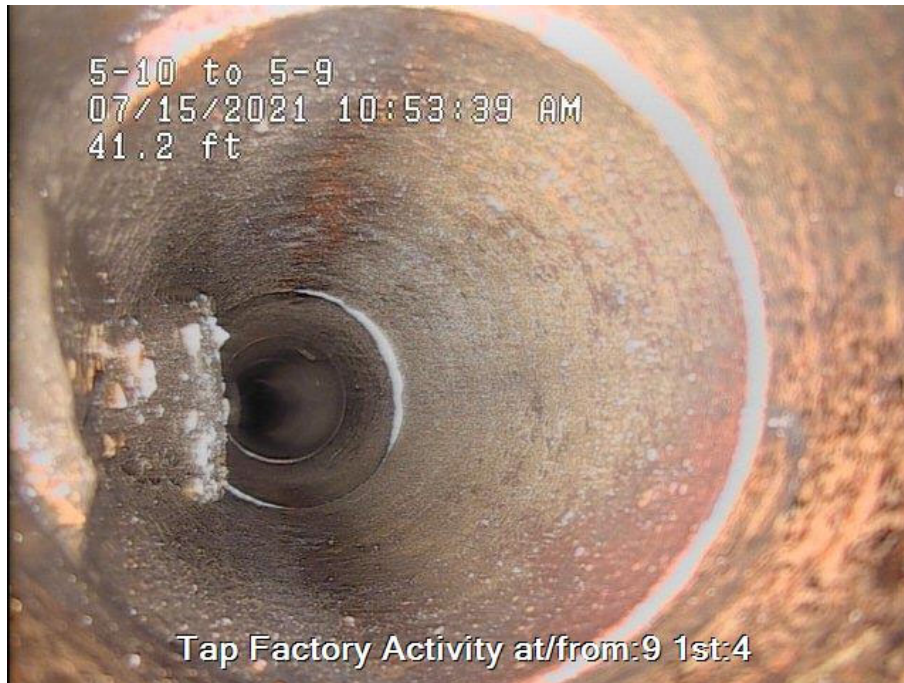
Example: Factory Tap - Intruding on Pipe Area
