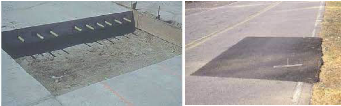
Figure 5 - Concrete and Asphalt Patches
