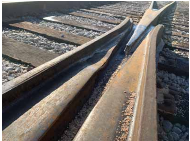
DEFORMED FROG WITH CRUSHED HEAD ALONG WING RAIL
