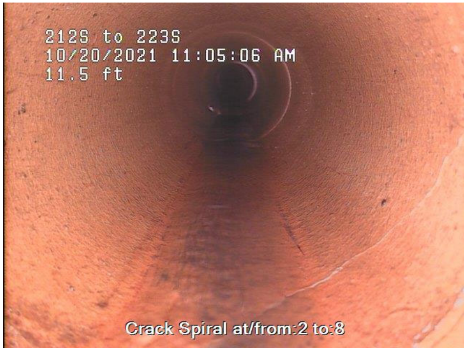
Example: Spiral Crack
