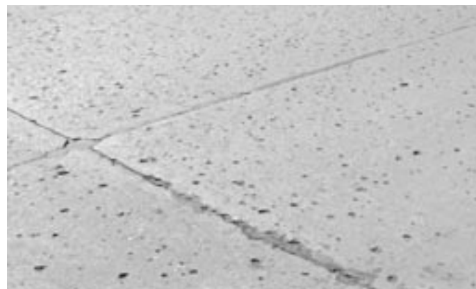
◀ Extensive pop-outs of large aggregate from surface. Pop-outs alone have not affected pavement serviceability.
