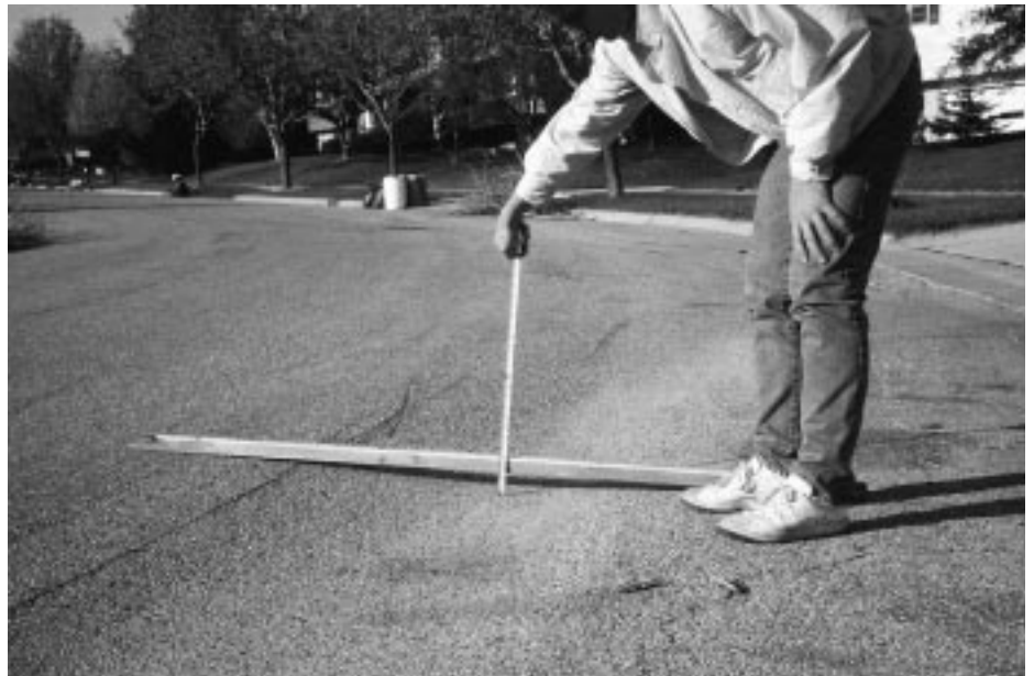
► Severe settling from utility trench.
