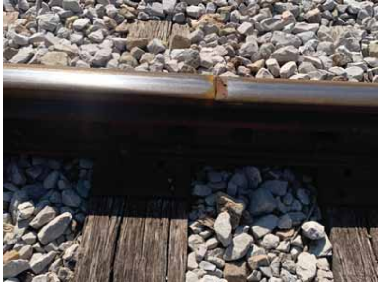
RAIL END BATTER (CHIPPED)
