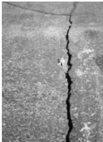
▲ Open crack – 1/2" or more in width.
