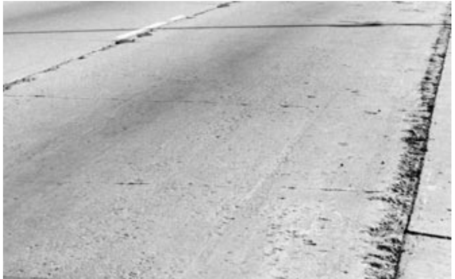
▶ Spalling along longitudinal joints.
