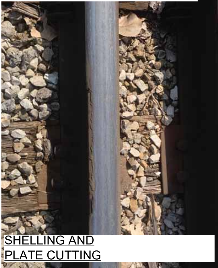
RAIL END BATTER (SMASHED)
