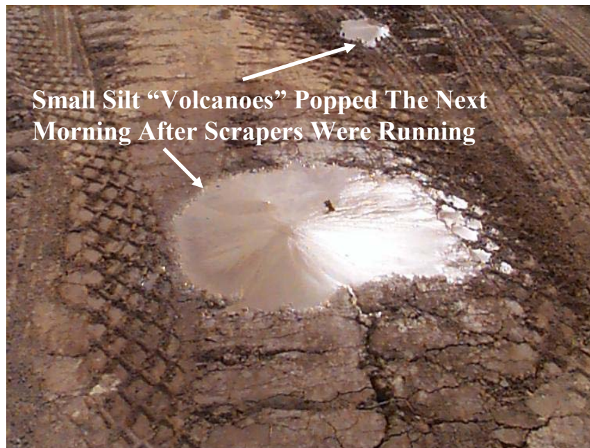
Figure 2. Repeated truck/equipment loads will draw moisture up to the surface of silty subgrade soils (pumping).
