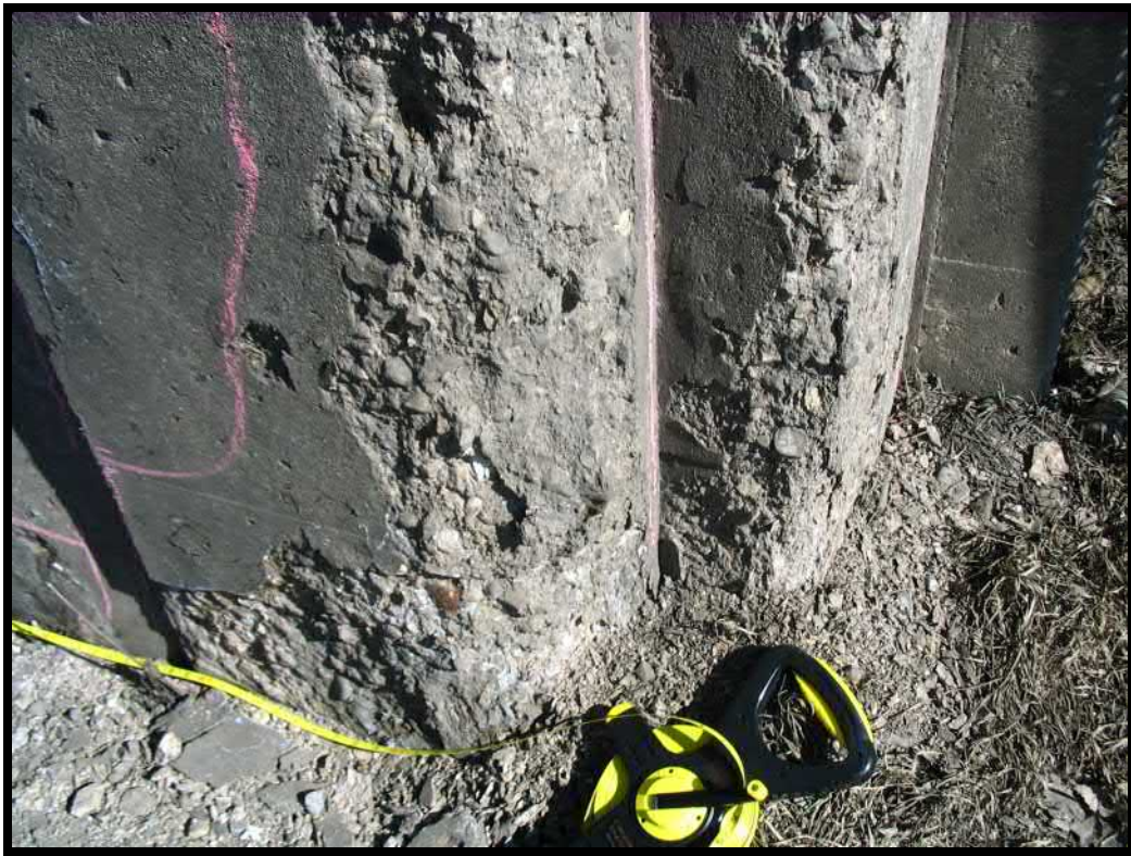
Photo 34. East Abutment—Spalling at south corner
