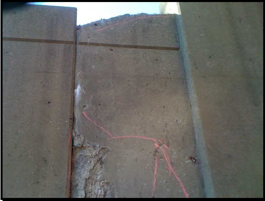
Photograph 31. Deep (greater than 5" in depth) spall at the top of the third step of the southwest wingwall
