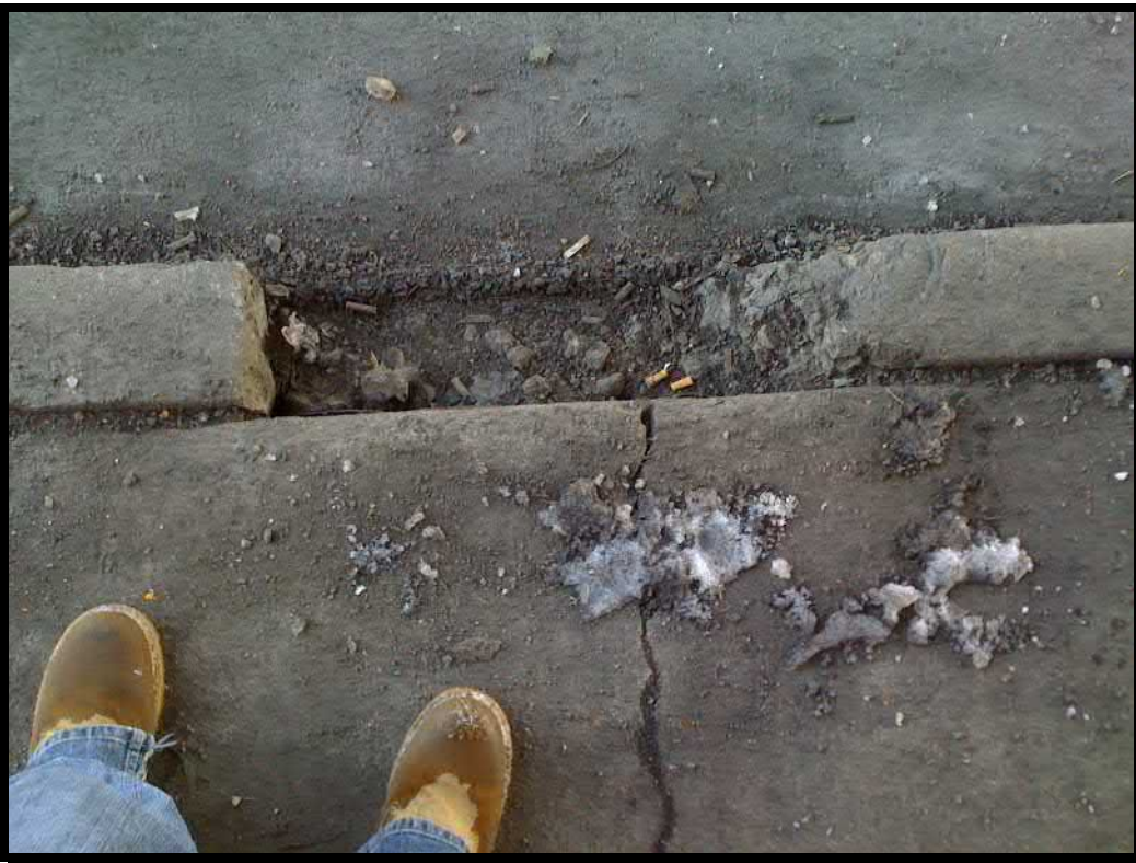
Photo 58. Cracks in sidewalk and chunks of curb missing below UPRR bridge
