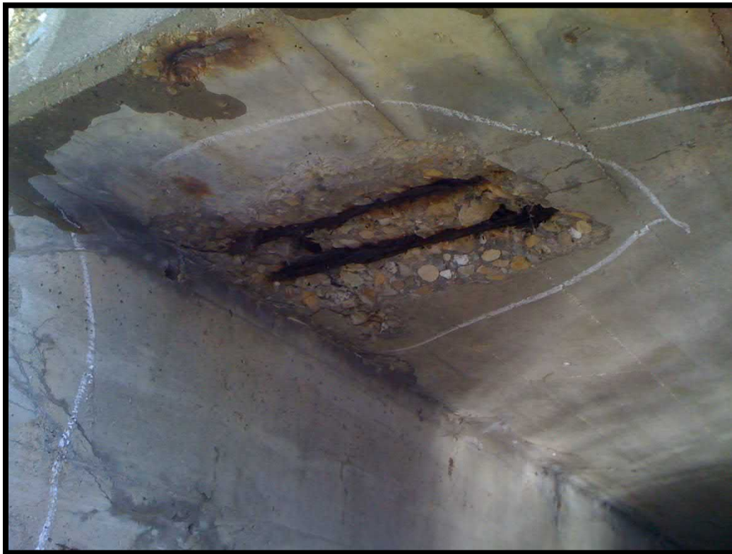
28. Exposed reinforcement at structure's west end, top slab
