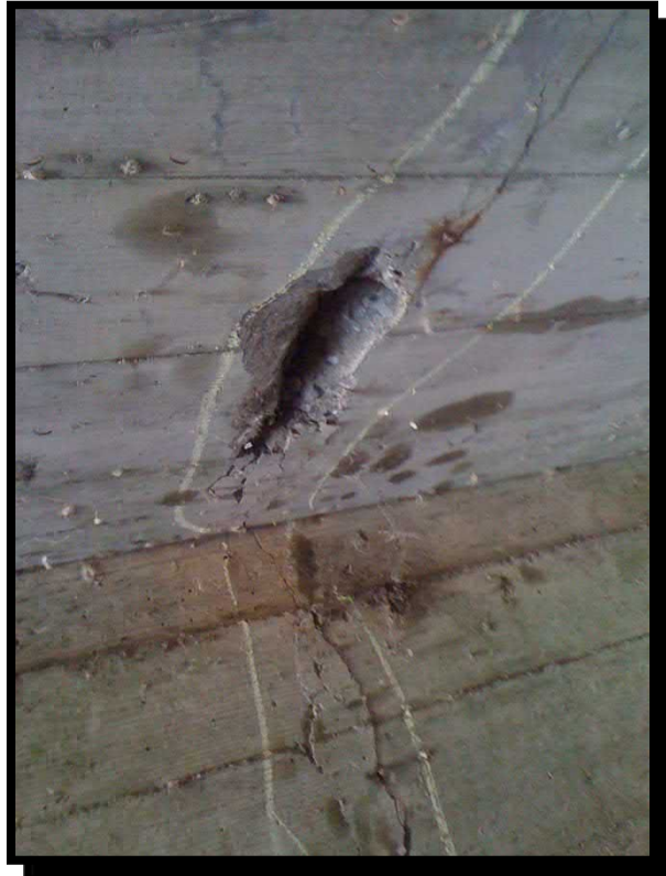
9. Delaminated and spalled top slab with exposed reinforcement
