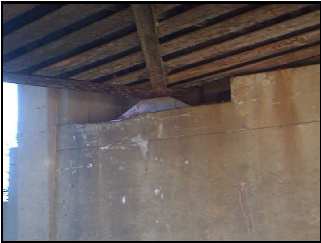
Photograph 20. Spall at top of the east abutment in front of north bearing seat
