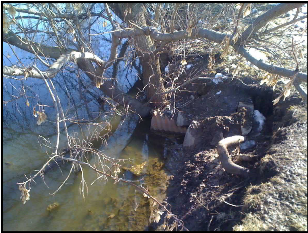
6. East end of dual drain pipes feeding pond overflow into east end of culvert
