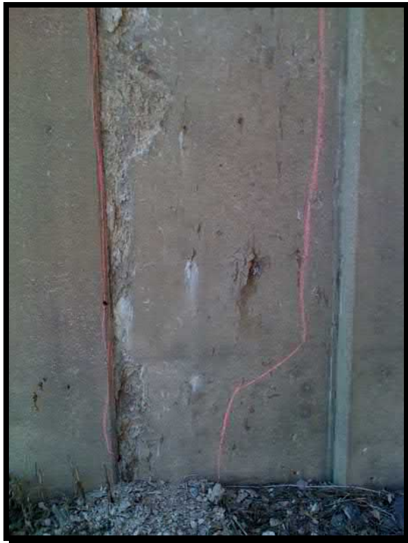
Photograph 30. Spalled and delaminated area in the third step of the southwest wingwall
