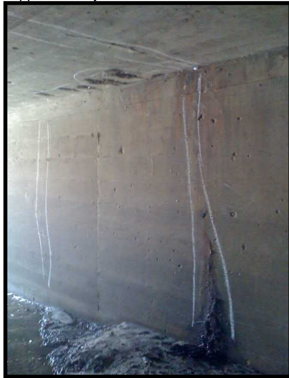
16. Open map cracks with moisture and rust located approximately 21 feet into the culvert from the east end
