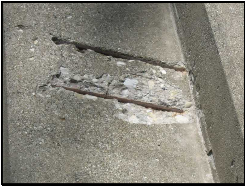
Photo 38. East Abutment–Exposed reinforcement
