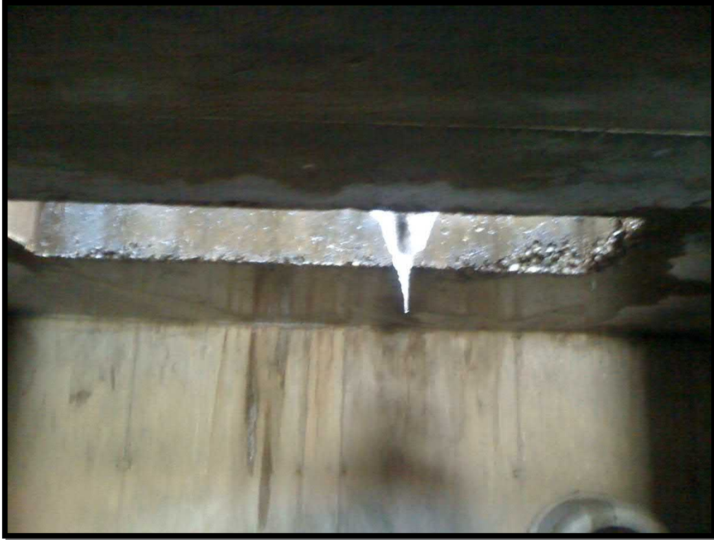
9. Inside view of inlet drain grate in top slab of west end culvert
