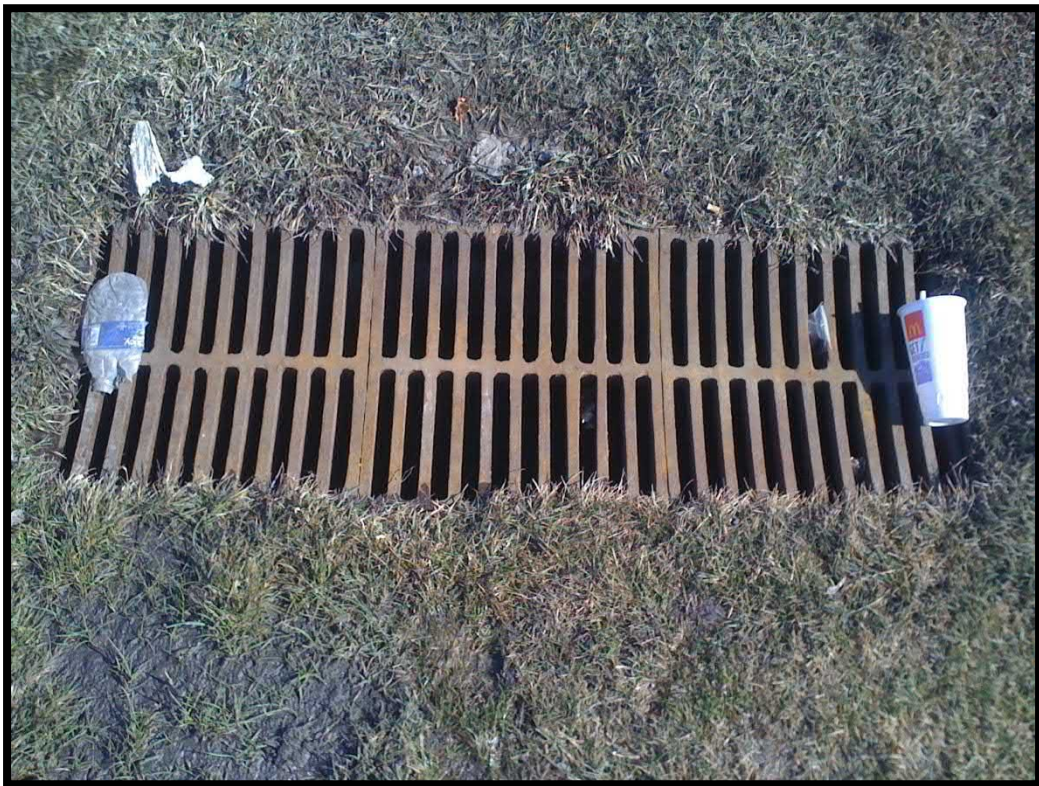
10. Outside view of inlet drain grate in top slab of west end of culvert
