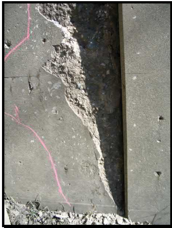
Photo 40. Southeast Wingwall–Spalled section
