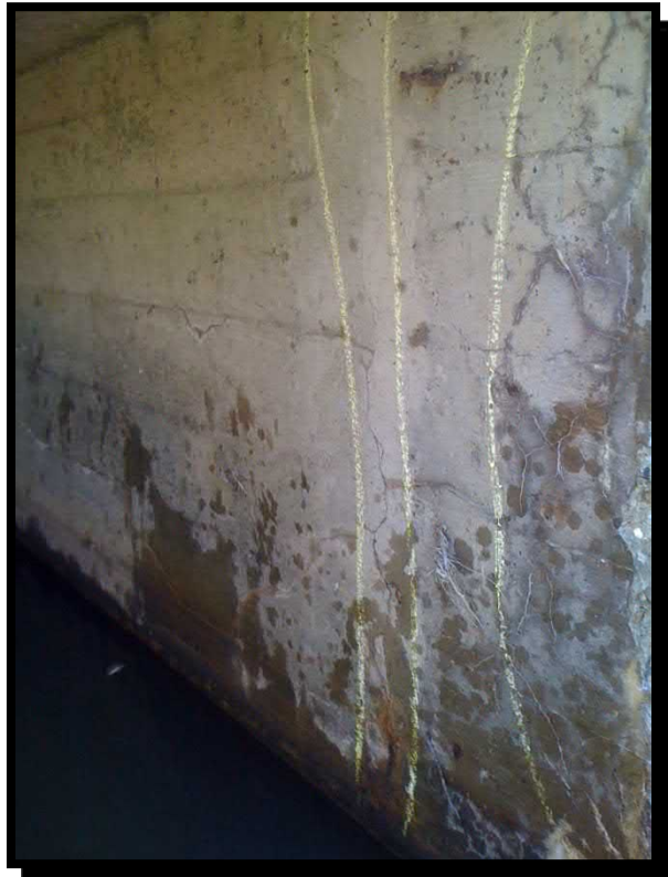
10. Open cracks with efflorescence, typical of three locations along walls
