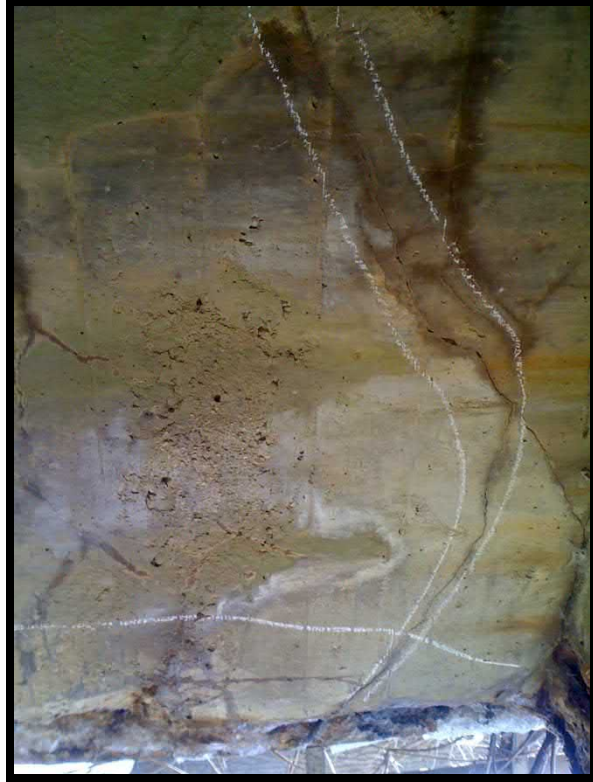
29. Open cracks and spalls propagating from west headwall
