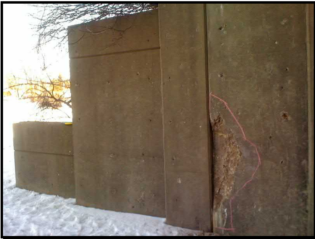
Photograph 26. Deep (greater than 5" in depth) spall in the northeast wingwall.
