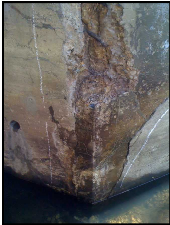
26. Delamination at corner of northwest wingwall
