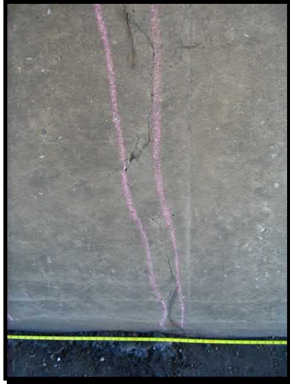
Photograph 19. Full height open crack on front face of the east abutment, typical of four locations
