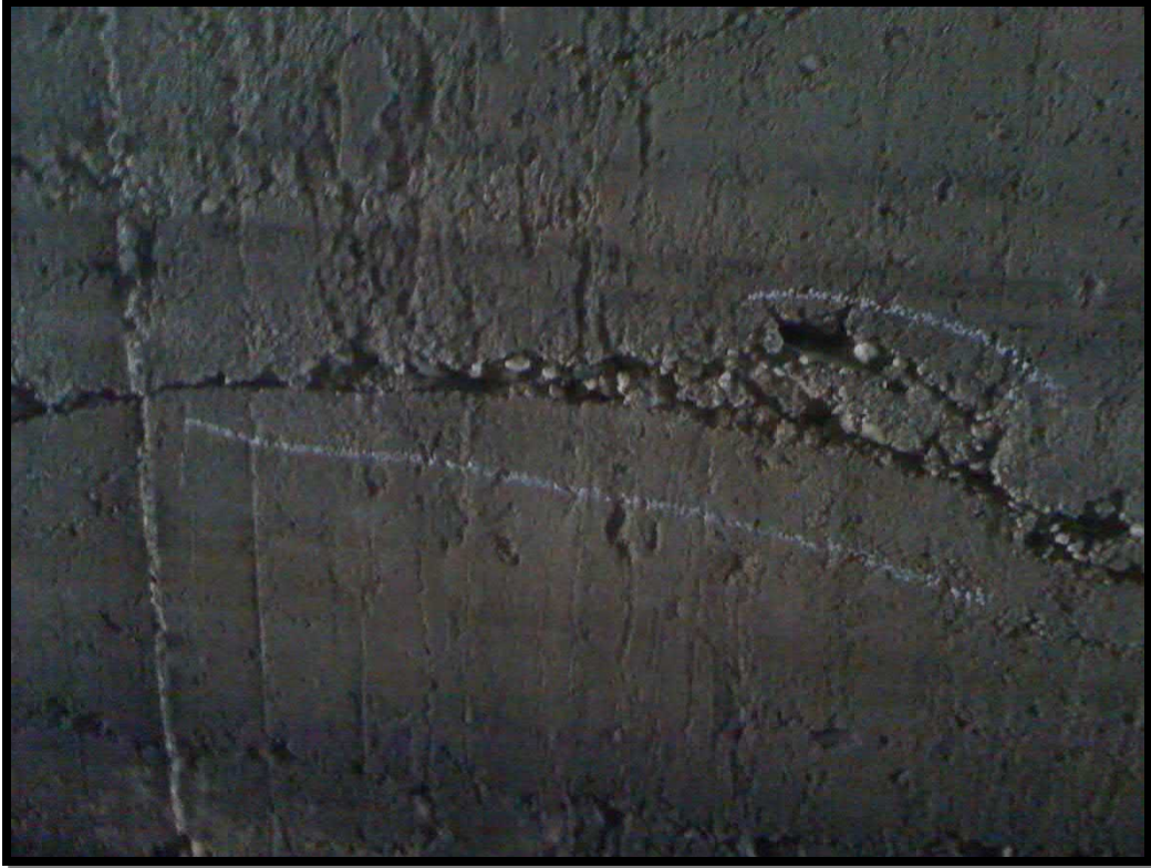
19. Open crack with spalls, typical of multiple locations on west barrel walls
