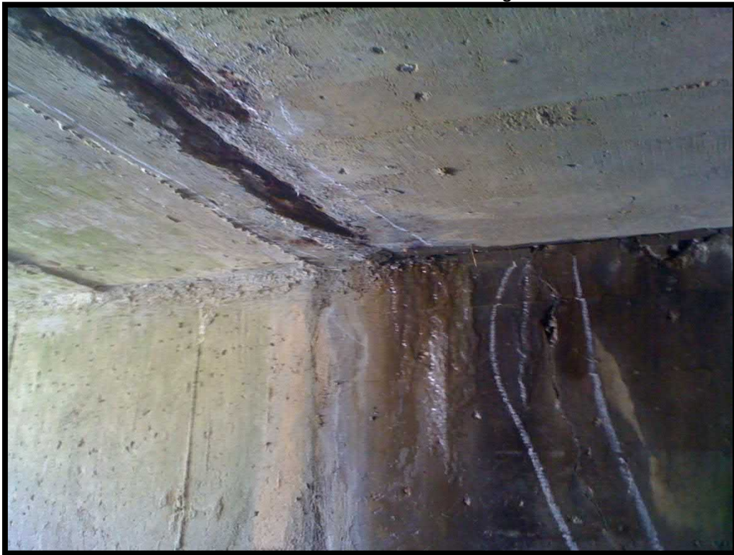
14. Exposed reinforcement and open map cracks located approximately 17 feet into culvert from the east end
