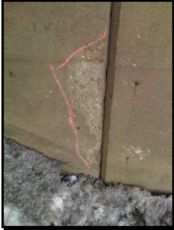
Photograph 29. Shallow (less than 5" in depth) spall in the northwest wingwall
