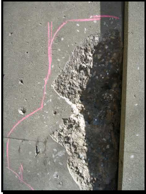
Photograph 27. Deep (greater than 5" in depth) spall in the southeast wingwall
