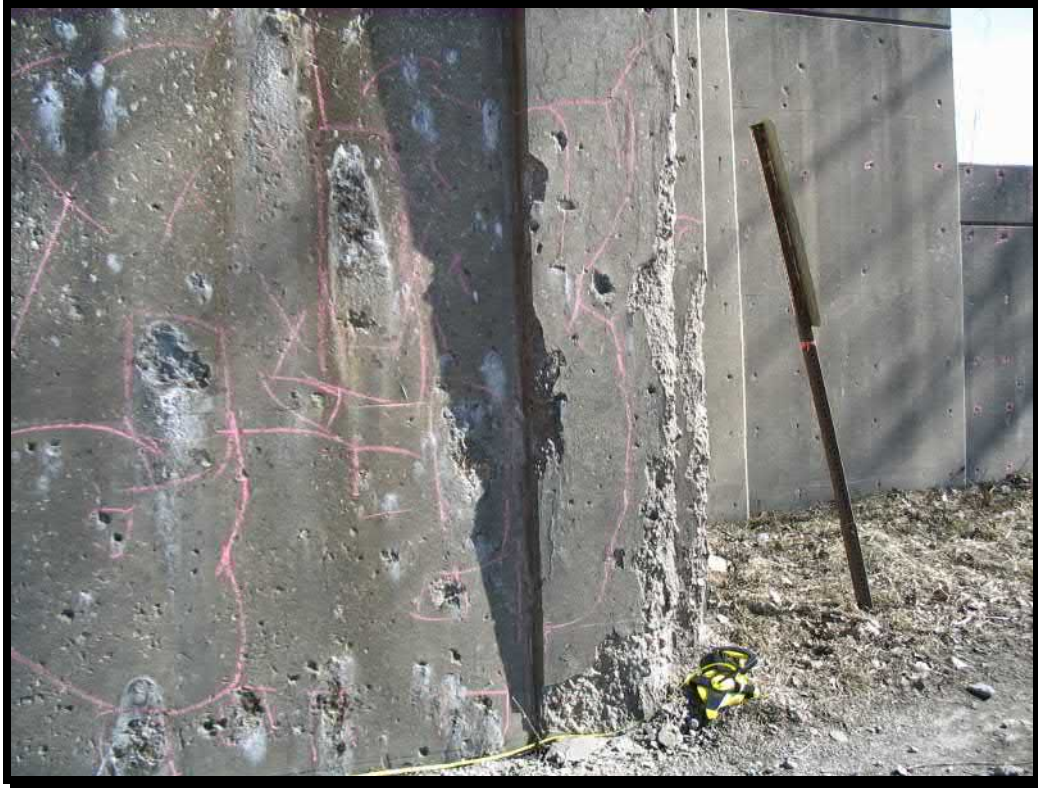
Photo 35. East Abutment—Spalling at south corner
