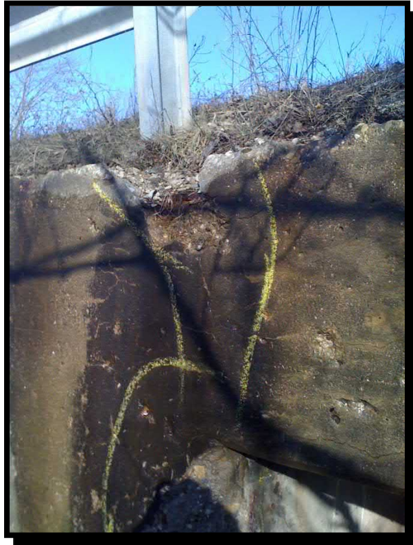
15. Cracks and spalls at north corner of west headwall
