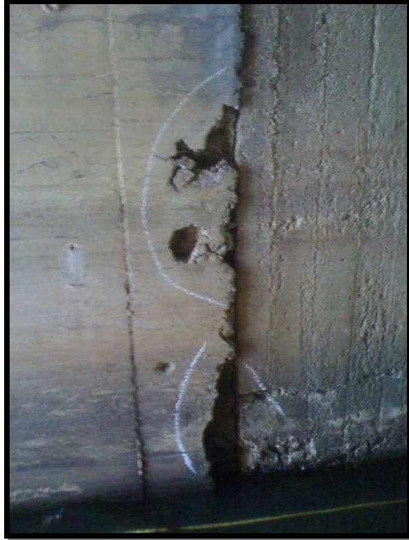
23. Spalls in the north wall around construction joint approximately 84 feet into the culvert from the east end
