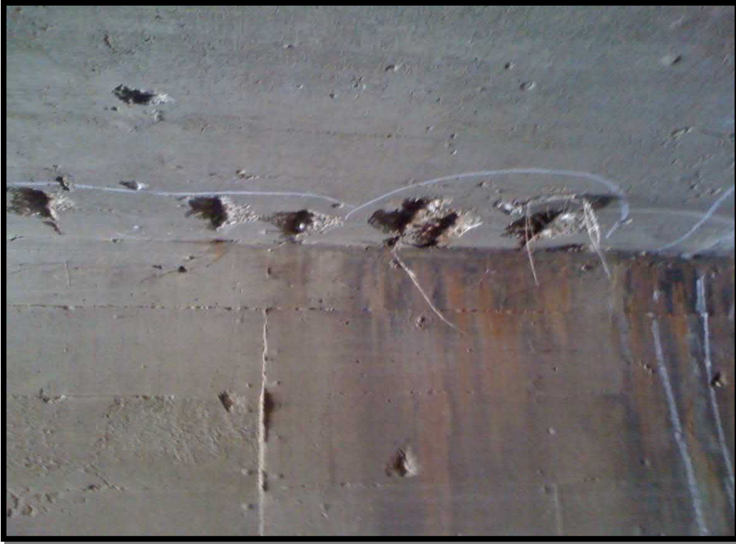
21. Group of spalls with exposed reinforcement located approximately 20 feet into the culvert from the east end
