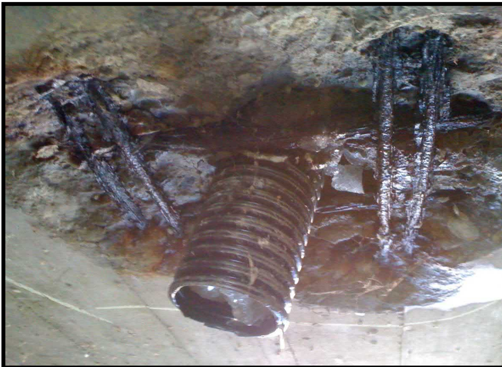
18. Hole in top slab with exposed reinforcement and protruding drain pipe
