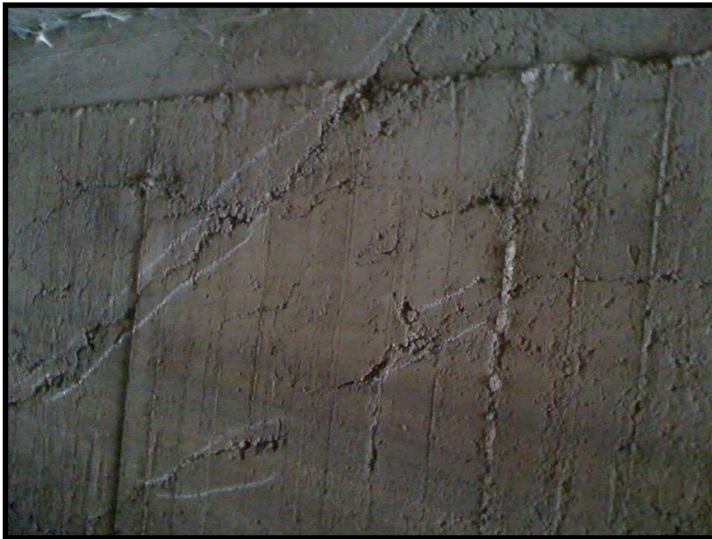
18. Hairline cracks, typical throughout west barrel walls
