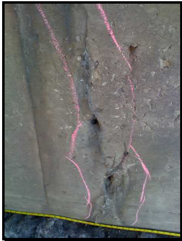
Photograph 22. Spalled area, typical of approximately 2% of the front face of the west abutment
