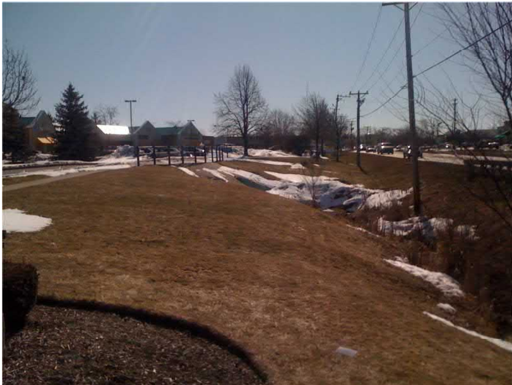
12. Drainage ditch with dense plant growth leading from east end of culvert to dual pipe culvert under Private Drive.
