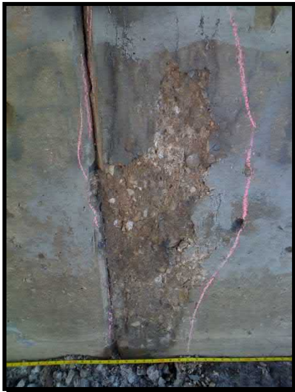
Photo 50. West Abutment—Spalling at construction joint
