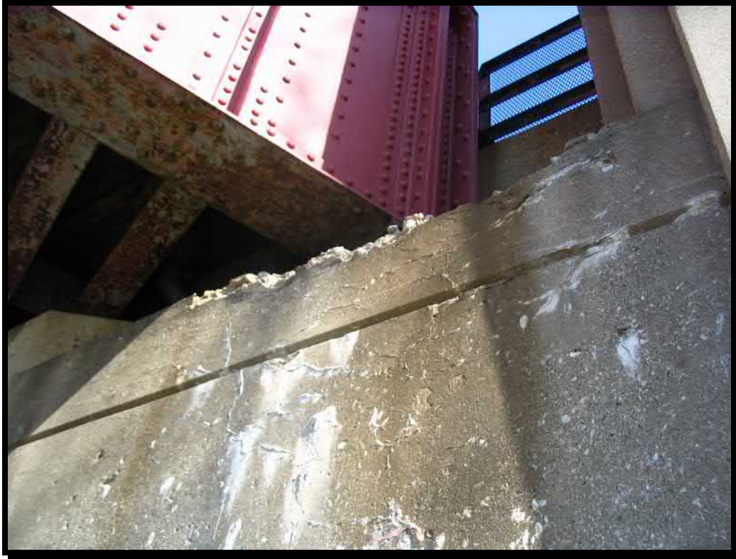
Photograph 21. Spall at top of the east abutment in front of south bearing seat
