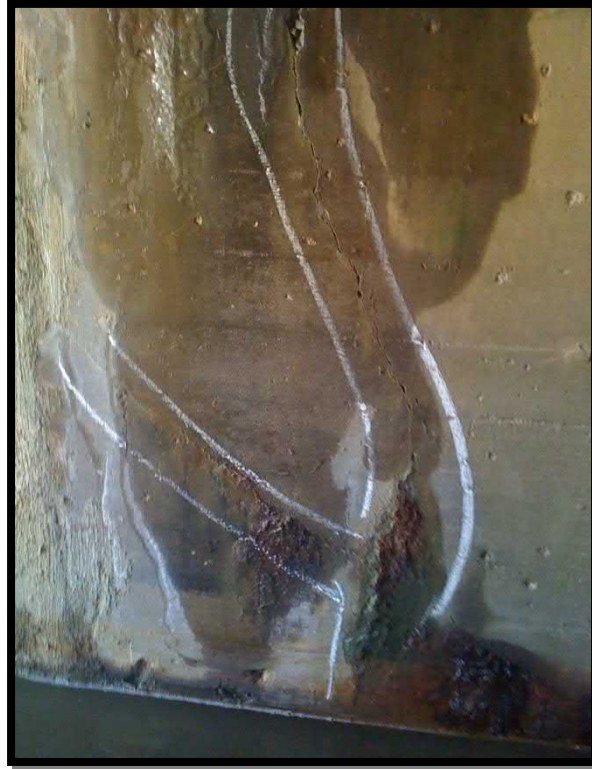
15. Open map cracks with moisture and efflorescence located approximately 17 feet into culvert from the east end
