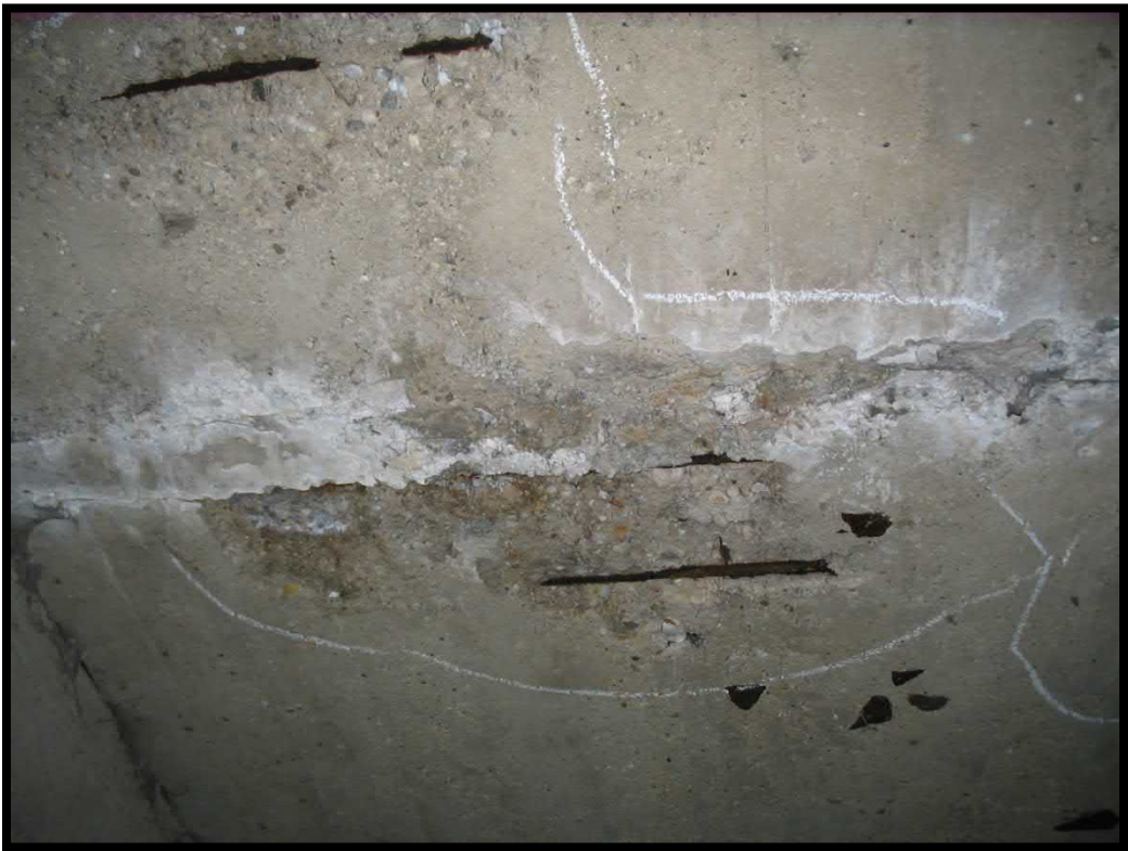
22. Delamination and exposed reinforcement on west barrel, top slab
