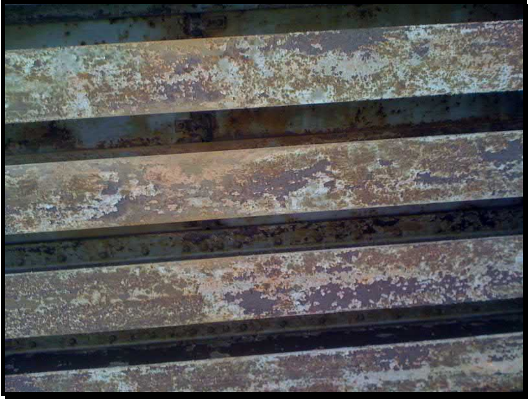
Photo 55. Floor beams depicting rust and paint peeling
