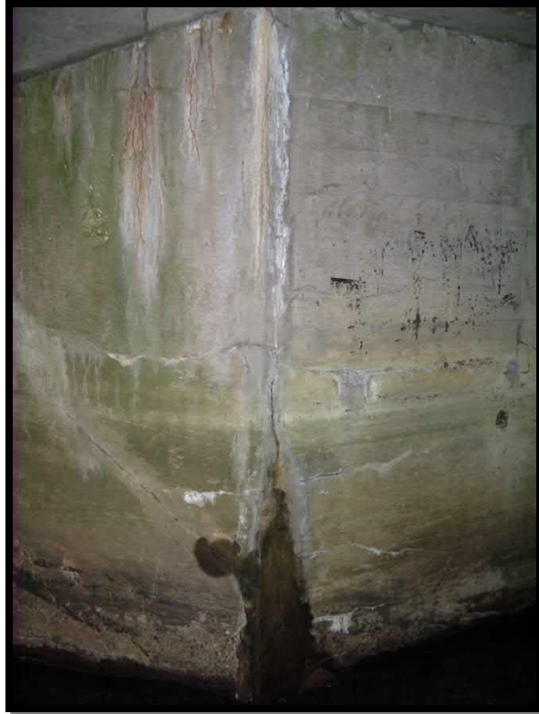
15. Open cracks, efflorescence, and spalls at the south transition wall bend
