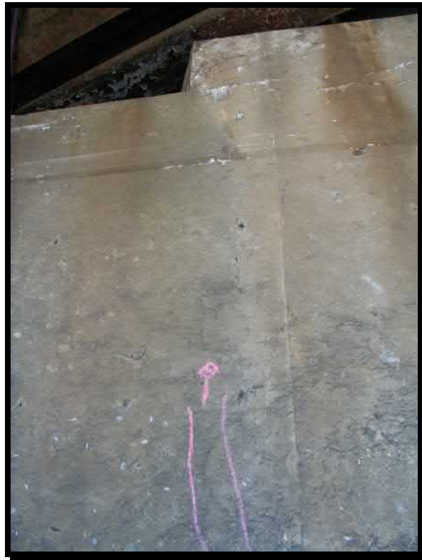
Photo 48. West Abutment-Full height crack
