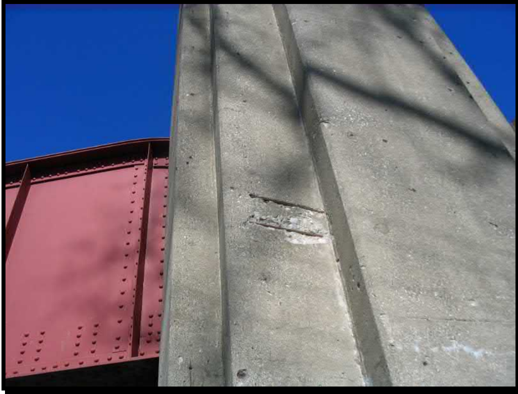
Photo 37. East Abutment–Exposed reinforcement
