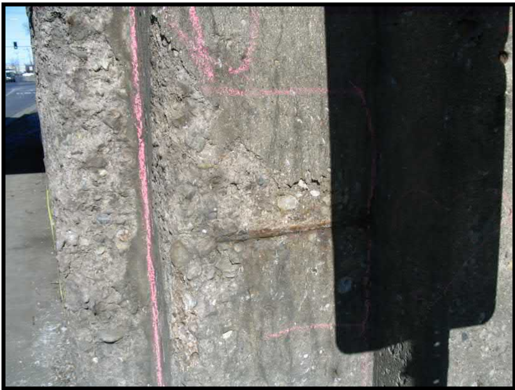
Photo 36. East Abutment—Spalling at abutment side
