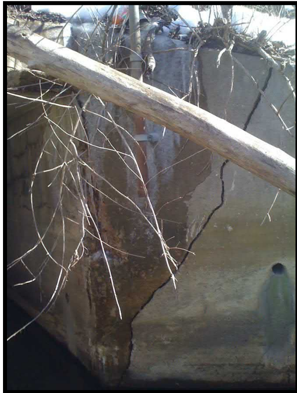
24. Full-height open crack in southwest wingwall
