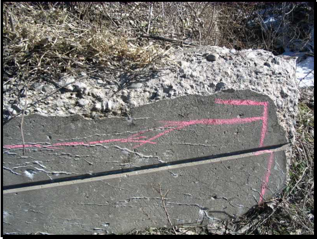
Photo 43. Southeast Wingwall–Spalled section
