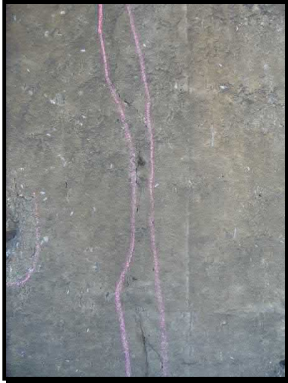
Photo 49. West Abutment—Full height crack
