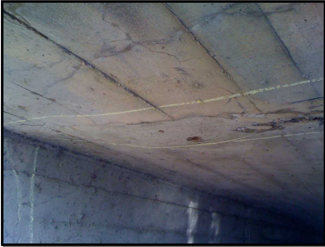
11. Delamination and map cracks with efflorescence, typical of three locations along walls
