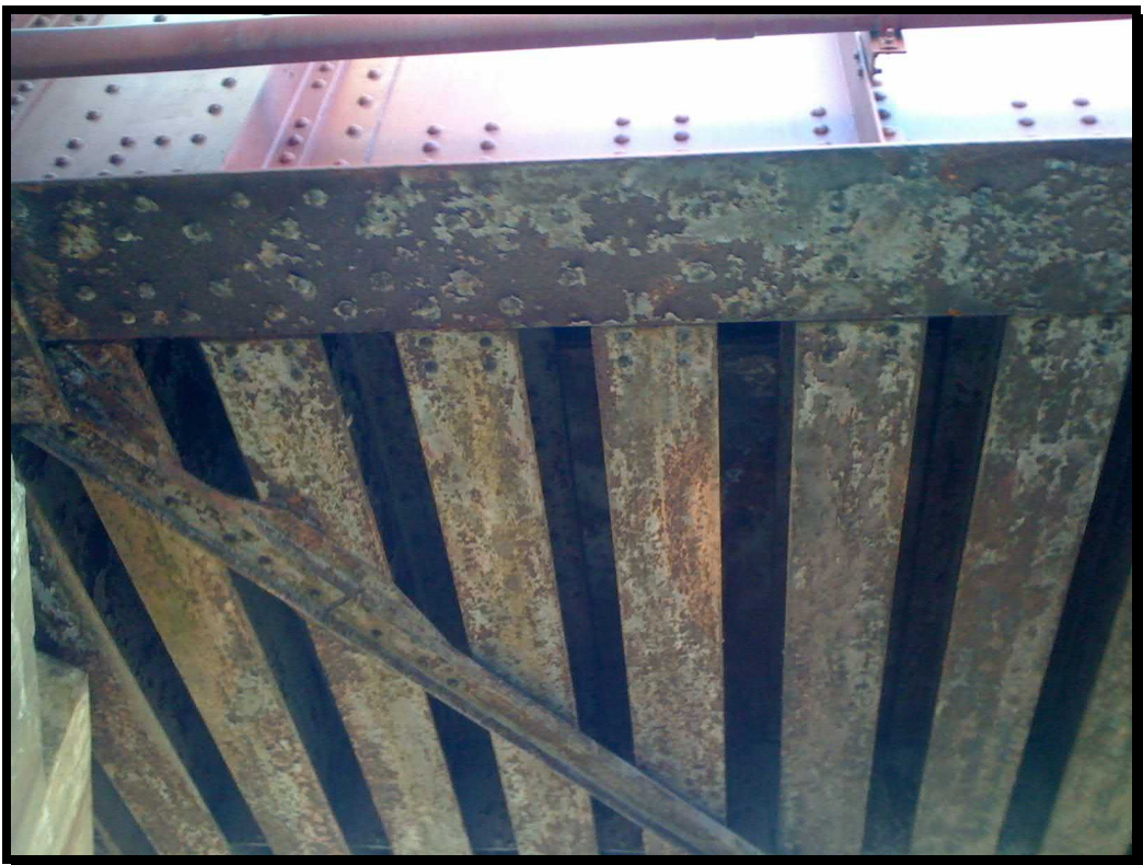
Photo 56. Girders depicting new paint on side with rust and paint peeling on base
