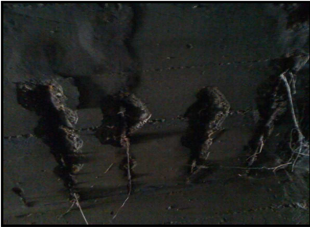
22. Group of spalls with exposed reinforcement located approximately 54 feet into the culvert from the east end
