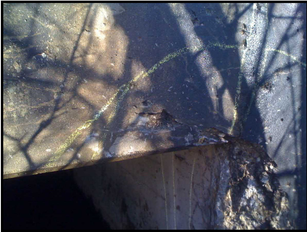
16. Cracks and spalls at south corner of west headwall
