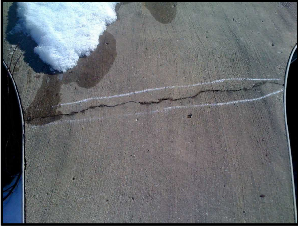
Photograph 9. Open crack in cast-in-place concrete headwall on west end of culvert
