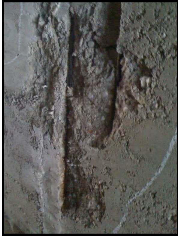
17. Delamination and exposed reinforcement, typical throughout west barrel walls
