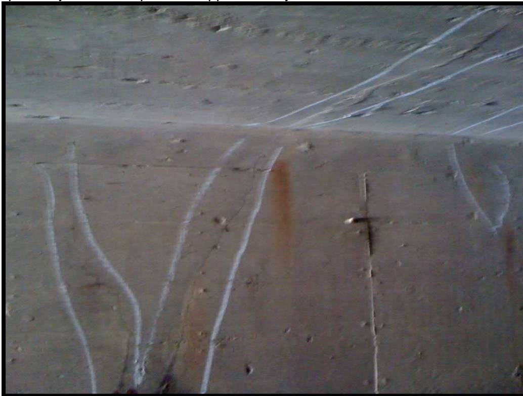
18. Open map cracks with efflorescence located approximately 26 feet into the culvert from the east end
