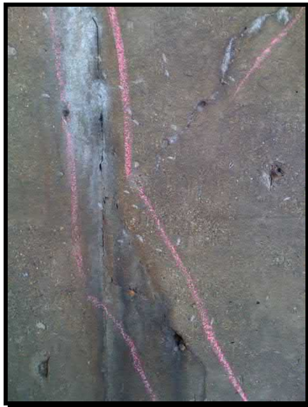
Photograph 24. Full height open crack with efflorescence, typical of three locations in front face of the west abutment
