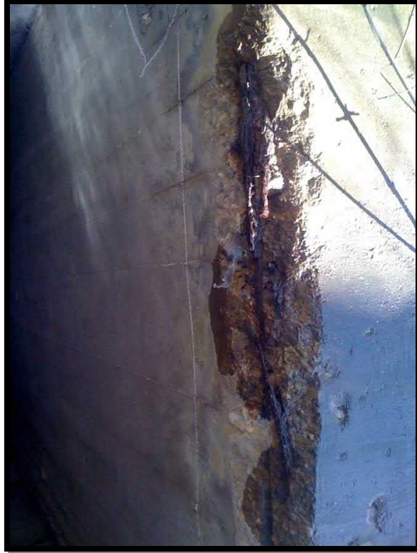
27. Delamination and exposed reinforcement at corner of southwest wingwall
