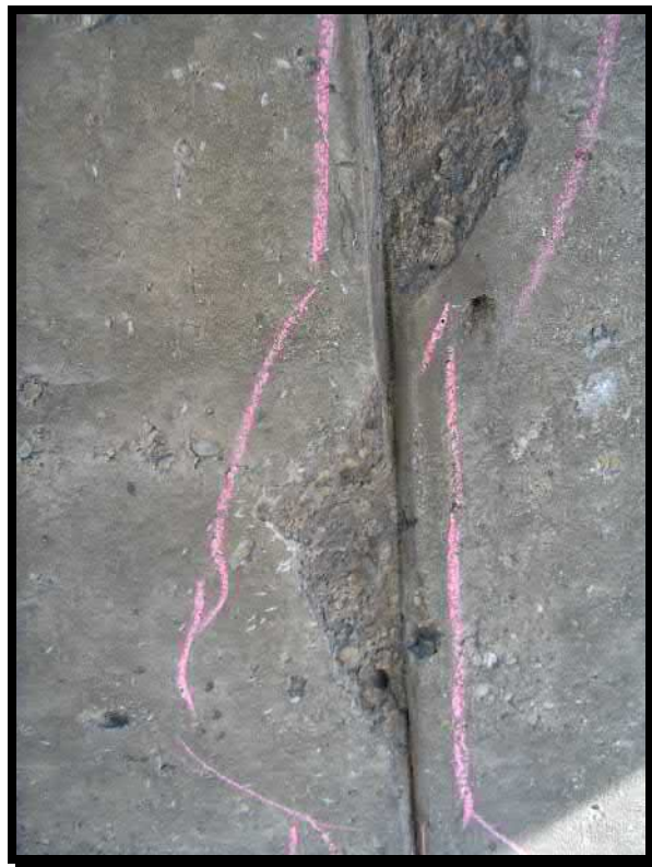
Photograph 16. Spalls along vertical construction joint in front face of the east abutment
