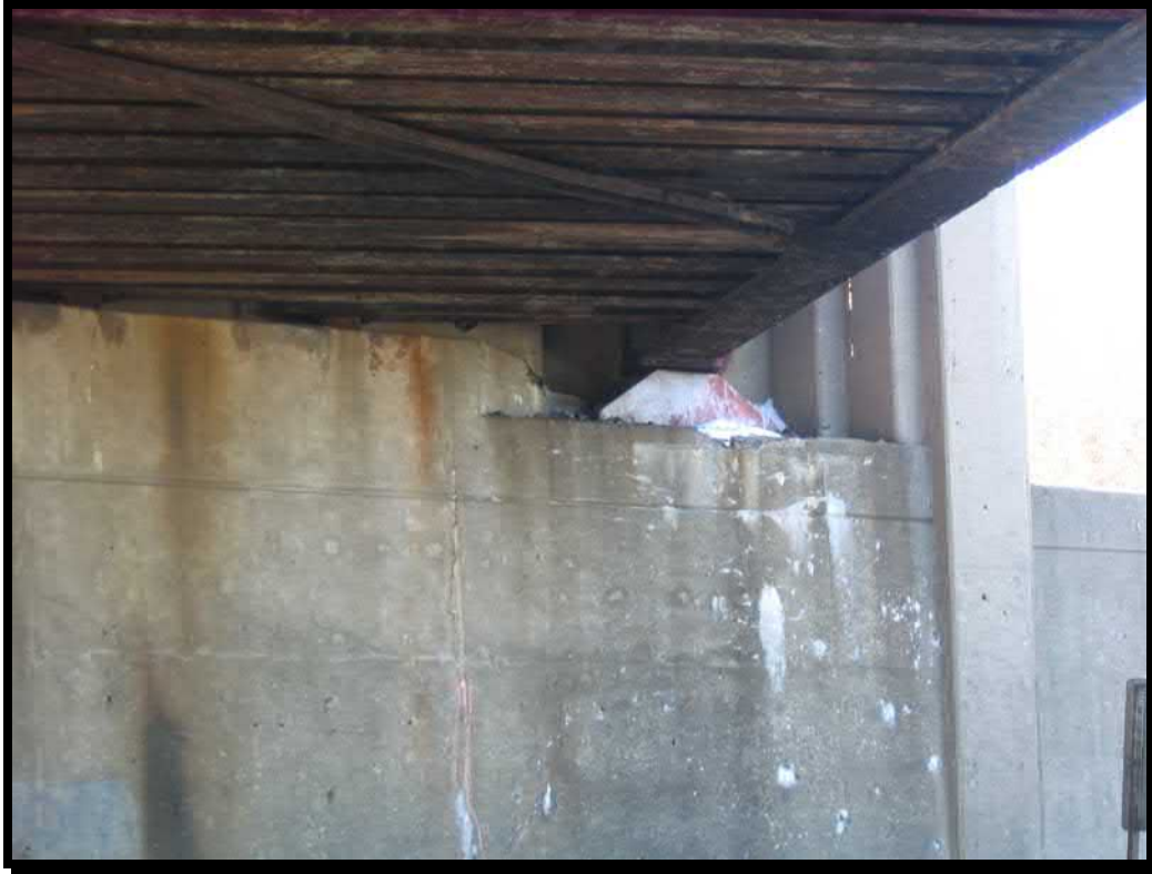
Photograph 25. Spall at top of the west abutment in front of north bearing seat
