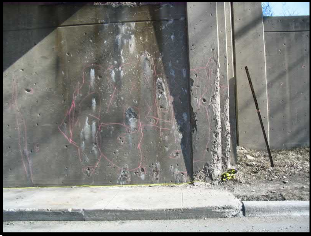
Photograph 17. Delamination and spalls with efflorescence, typical of approximately 15% of front face of the east abutment
