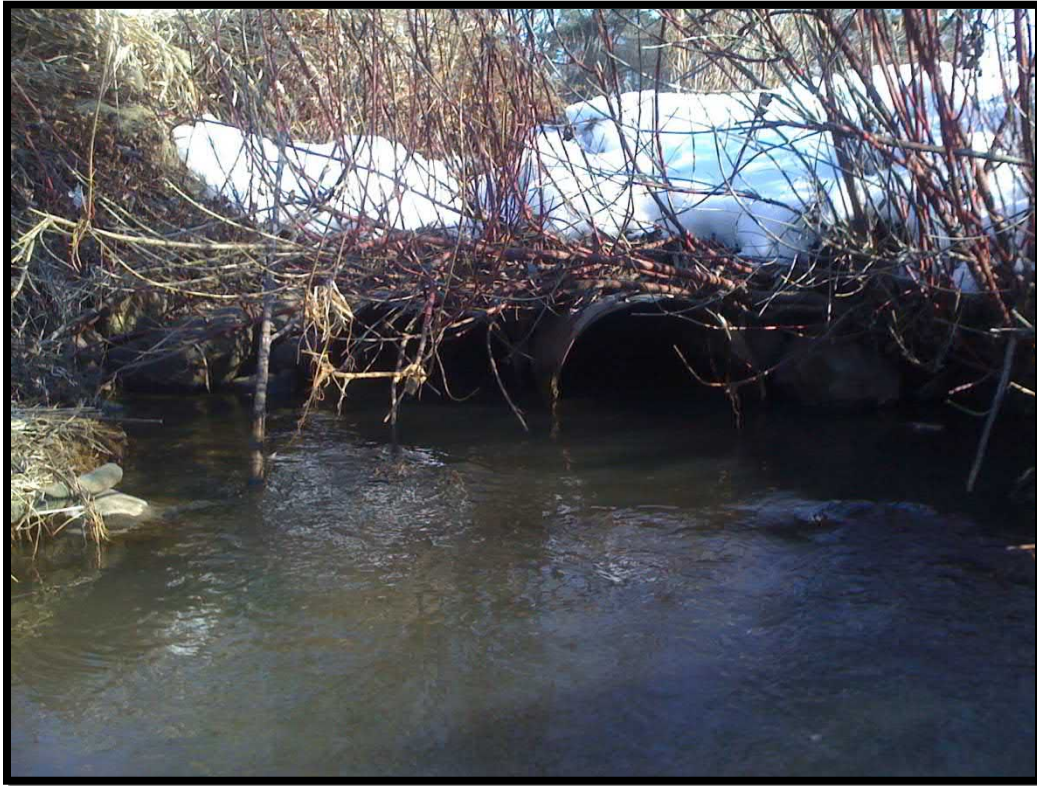
5. West end of dual drain pipes feeding pond overflow into east end of culvert
