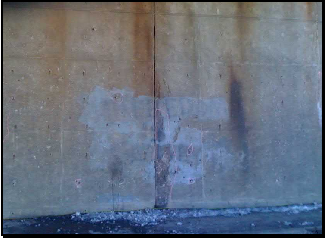
Photograph 23. Spalls along vertical construction joint in front face of the east abutment
