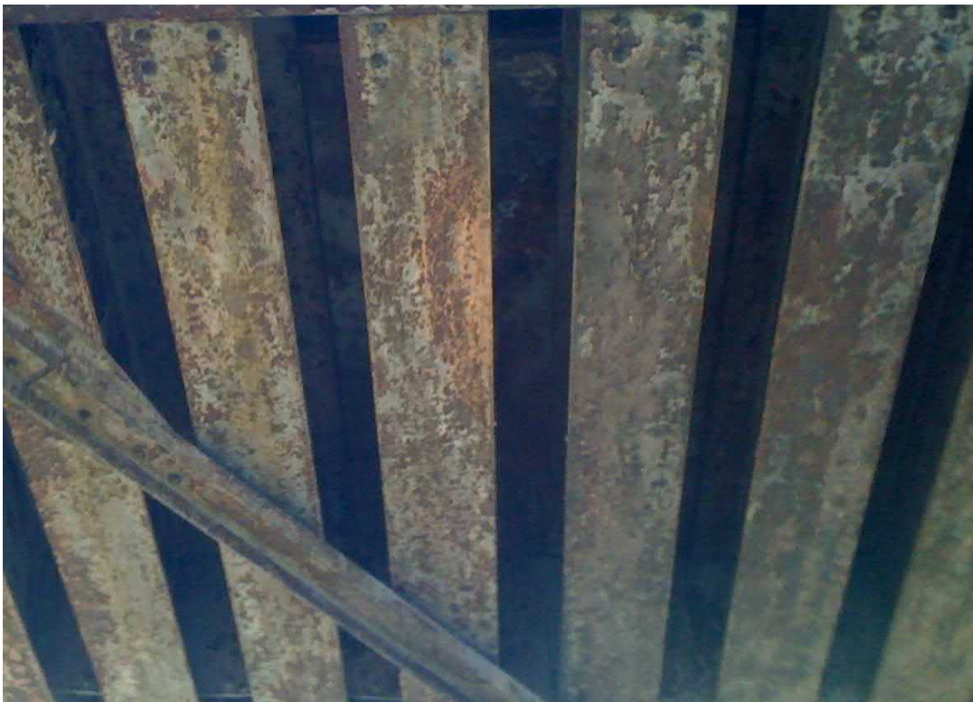
Photograph 12. Surface rust on steel floor plates (between beams), viewed from beneath the bridge
