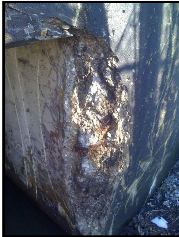
17. Spalls and open cracks at corner of southwest wingwall, typical of both wings
