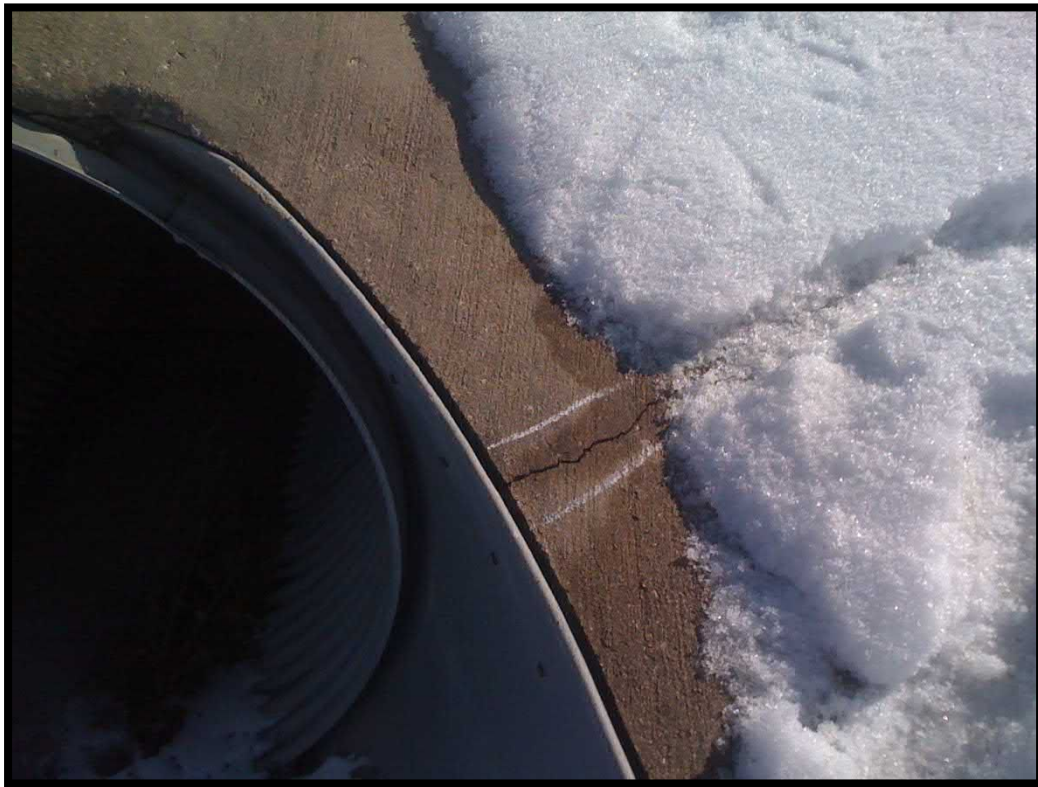
Photograph 8. Open crack in cast-in-place concrete headwall on west end of culvert
