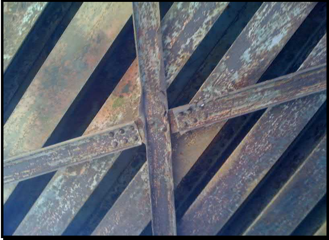
Photograph 15. Close-up view of damaged flanges on continuous leg of cross brace
