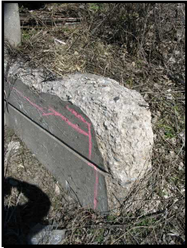
Photograph 28. Deep (greater than 5" in depth) spall in the first step of the southeast wingwall
