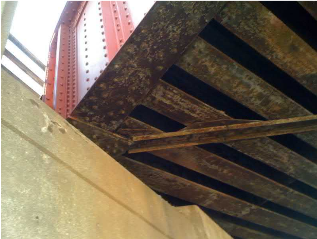
Photograph 13. Rust on bottom of bottom flange and recently painted outside face, typical of both exterior thru-girders
