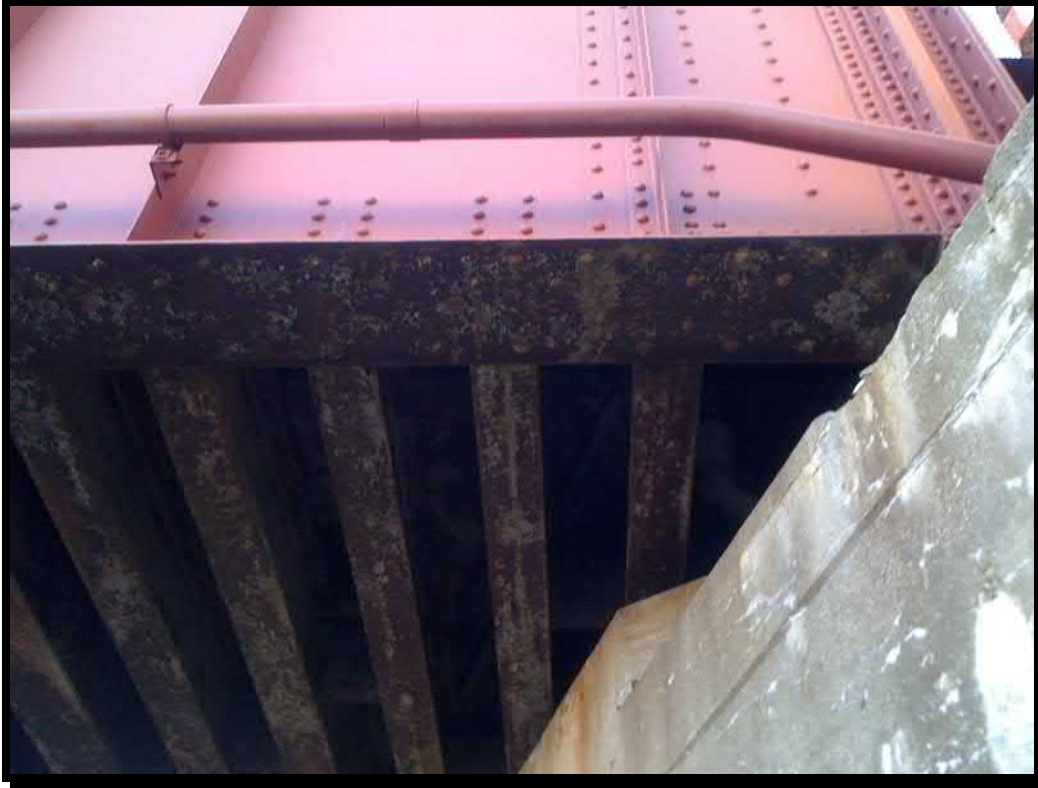
Photo 57. Girders depicting new paint on side with rust and paint peeling on base
