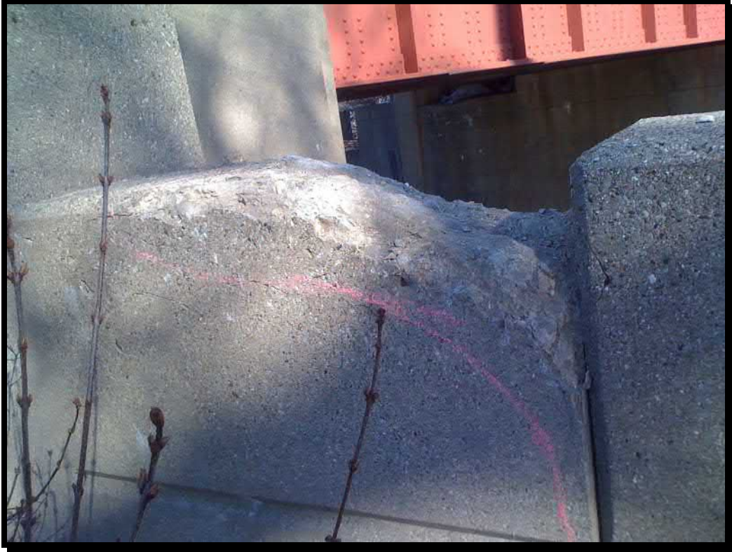
Photo 53. Southwest Wingwall spalling
