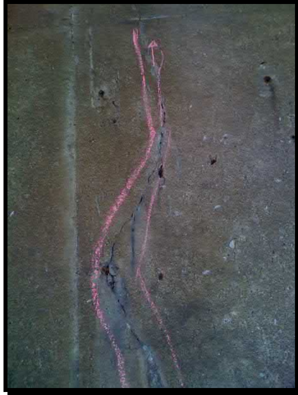
Photo 51. West Abutment–Full height crack
