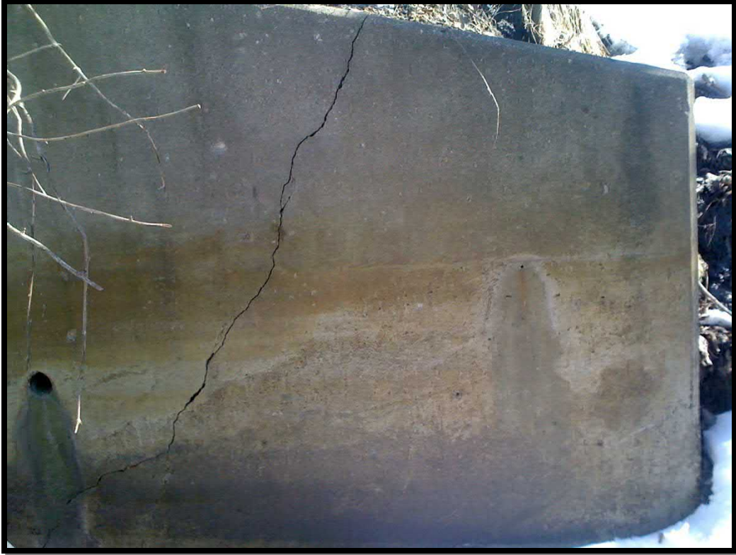
25. Full-height open crack in the northwest wingwall
