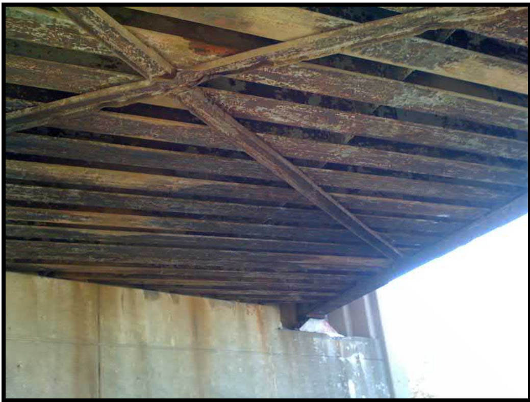
Photograph 14. Damaged flanges on continuous leg of "X-brace" near midpoint of brace
