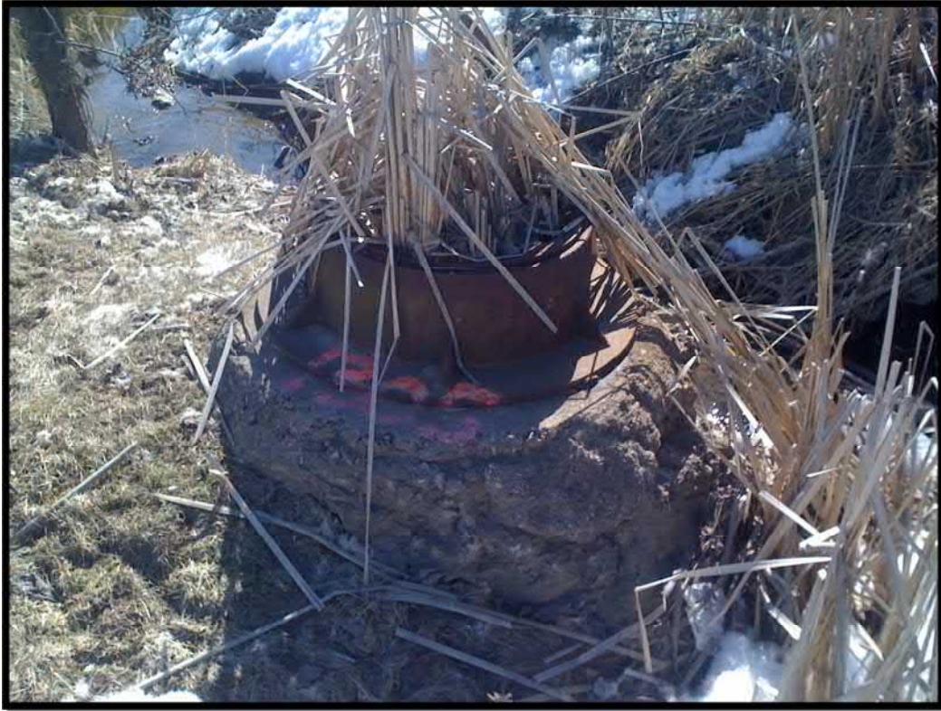
11. Clogged storm sewer intake near the southeast wingwall
