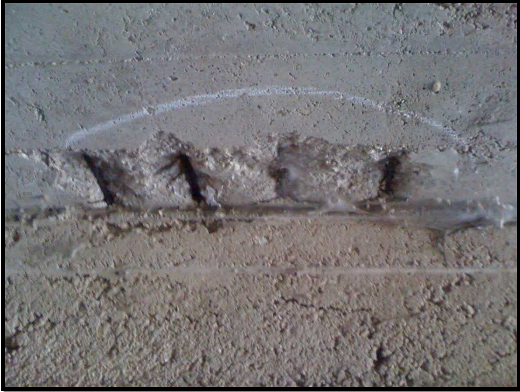
21. Exposed reinforcement on west barrel, top slab
