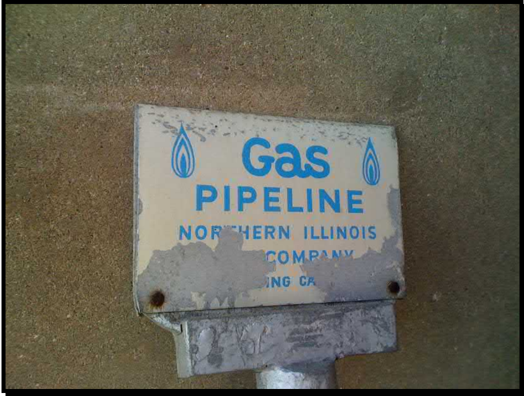
Photograph 9. Gas pipeline utility marker near southwest wingwall
