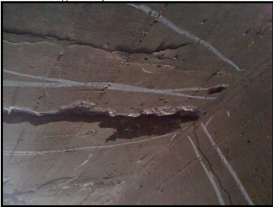
20. Delamination and map cracks in top slab at approximately 51 feet into the culvert from the east end
