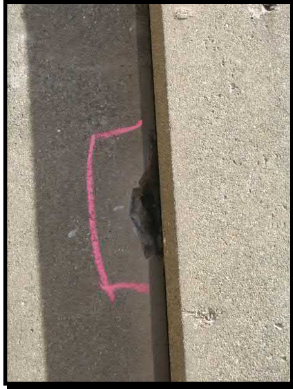
Photo 39. Southeast Wingwall–Spalled section
