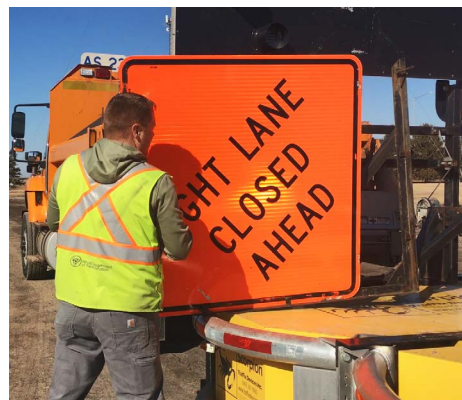
The ability to change signage with both feet on the ground reduces safety hazards.
