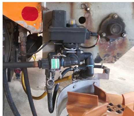
The three-way valve is controlled from inside the cab.
